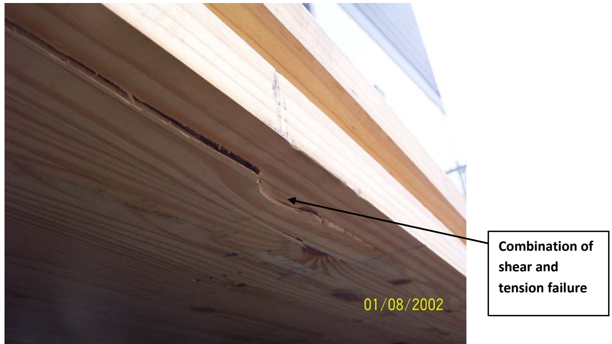
Figure 11c. Ultimate Failure – “Unzipping” of Lower Side of Groove
