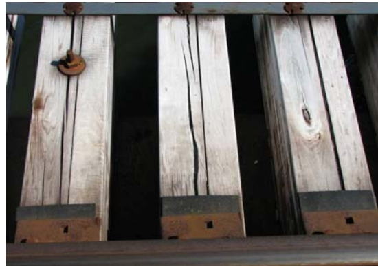
Figure 4: Crack development near lifting bolt
