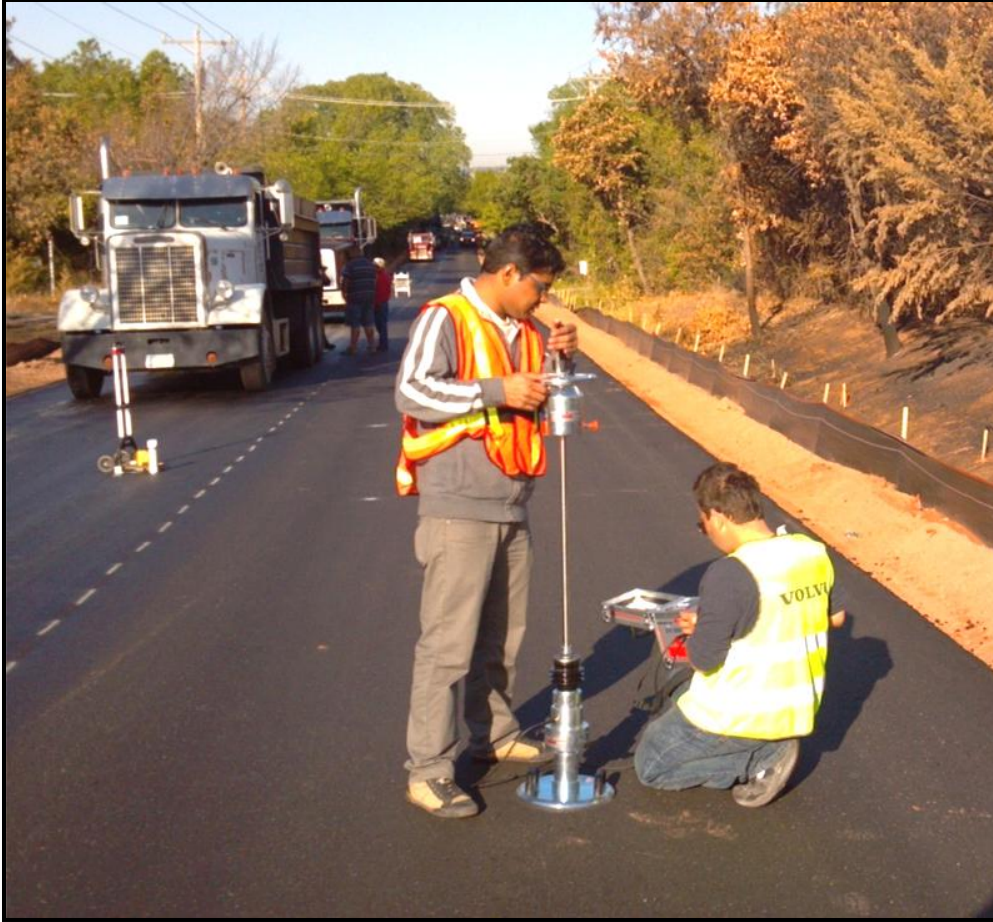
Figure 4. LWD Testing in progress at Apple Valley Road Project in Edmond, OK
