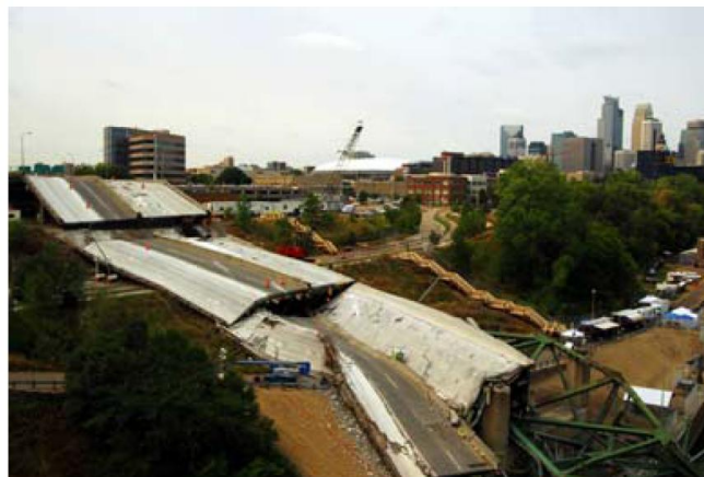
Figure 1.1. I-35W Bridge over the Mississippi River in Minneapolis collapsed.
