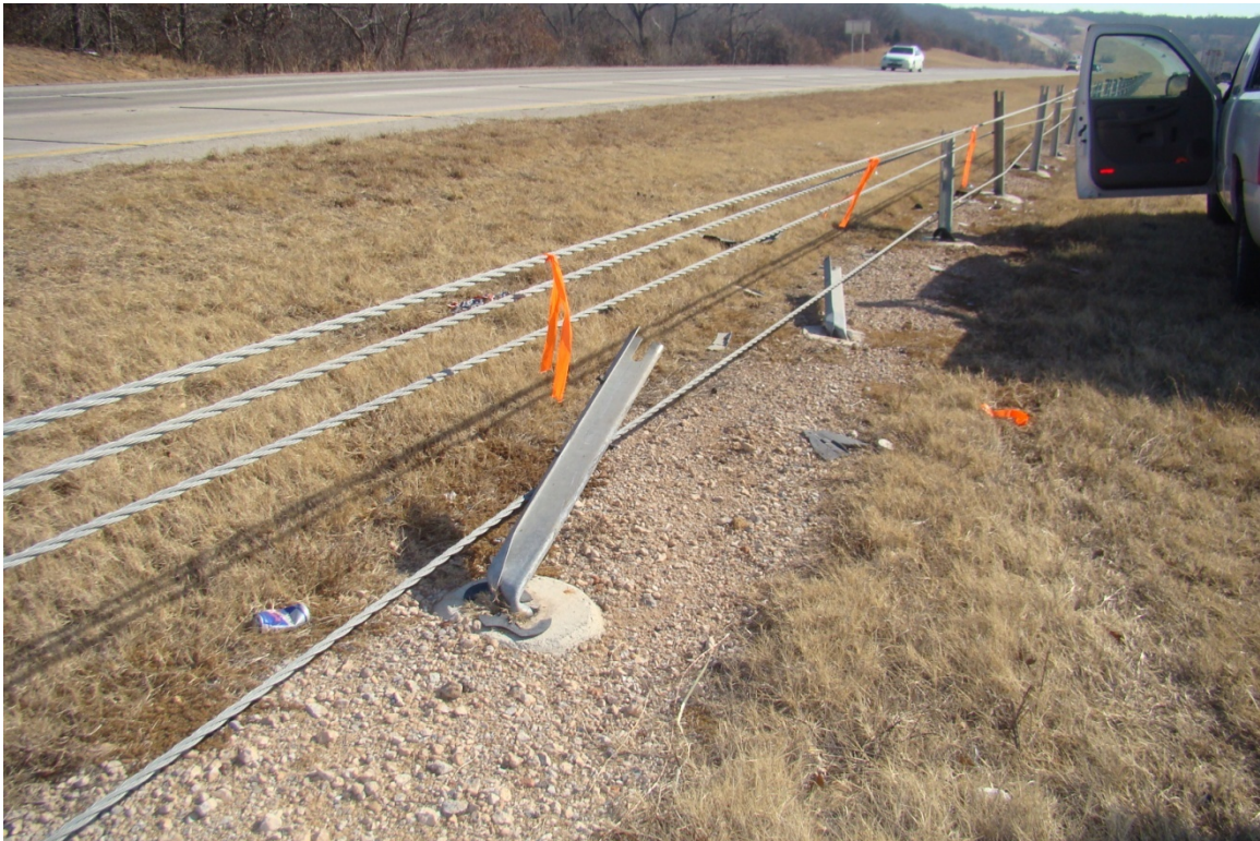
Figure 14 Typical Damage to Cable Barrier after Vehicle Impact
