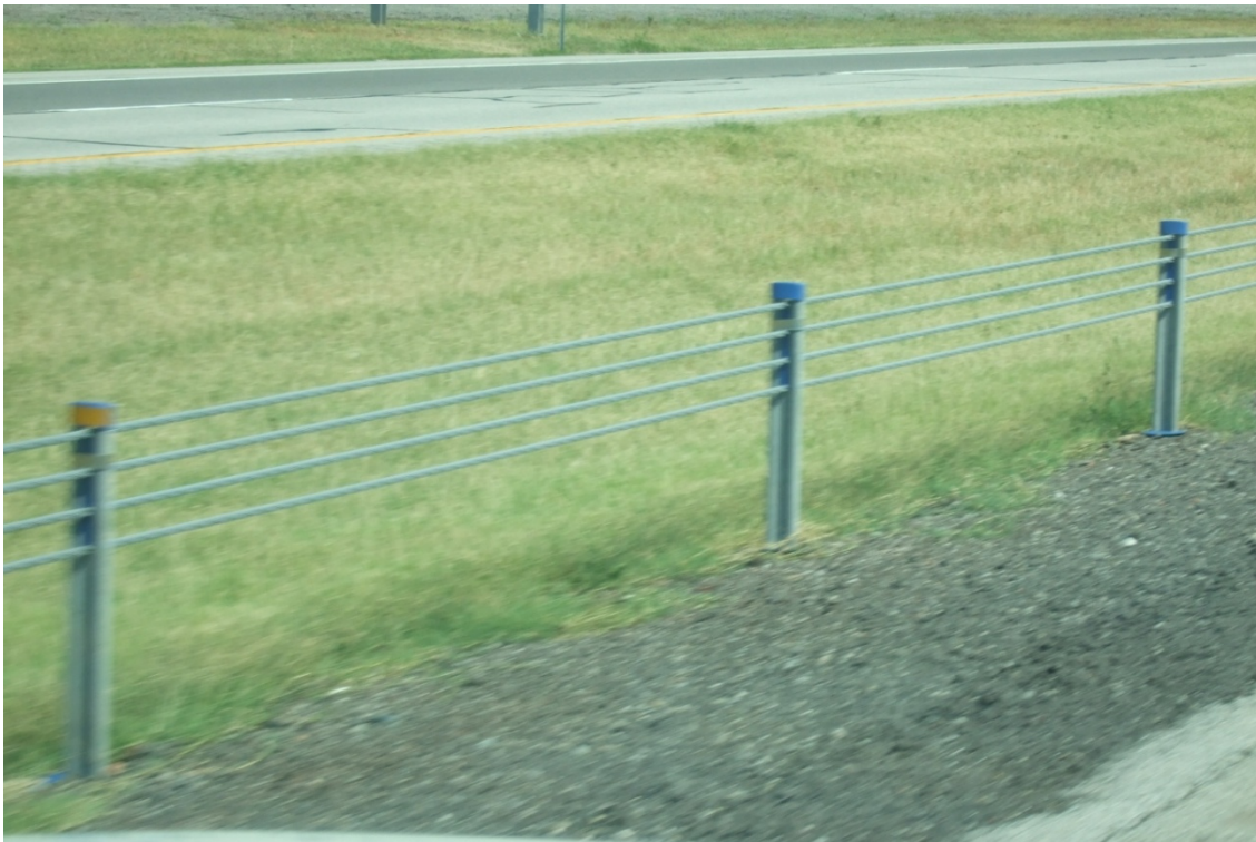
Figure 17 Blue Systems Safence
