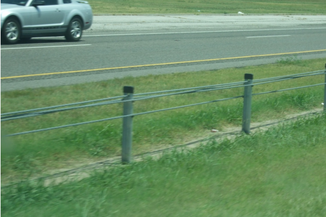
Figure 15 Brifen Wire Rope Safety Fence (WRSF)
