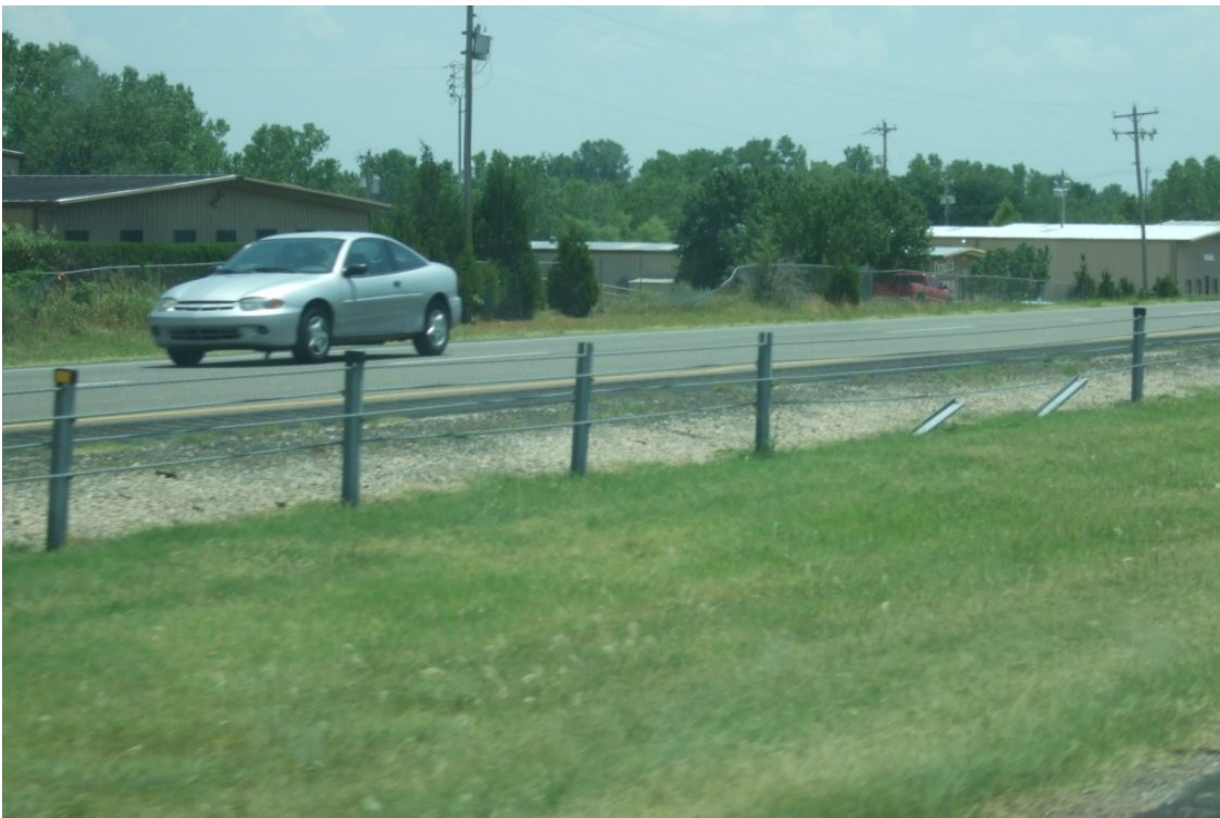
Figure 7 Damaged Cable Barrier on I-35
