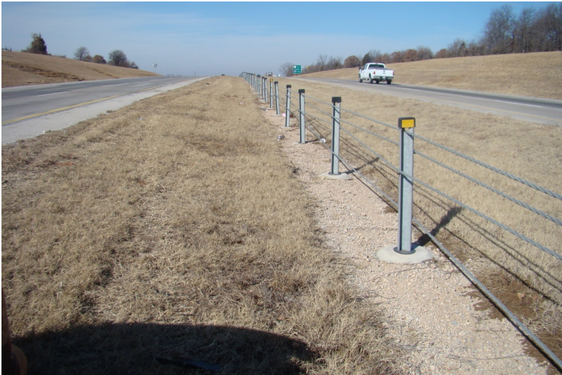
Figure 12 Cable Barrier installed in center of median
