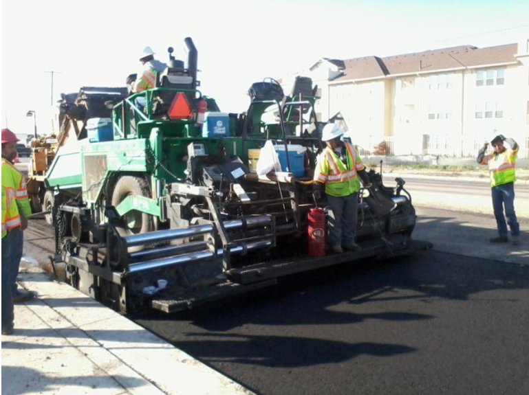
Figure 3.15 Placement of Evotherm ® Type C Mix on Foster Road, San Antonio, TX
