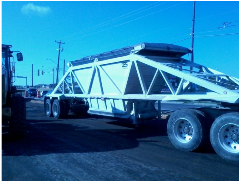
Figure 3.9 Placing the Evotherm ® Type B Mix on Foster Rd. in San- Antonio, TX
