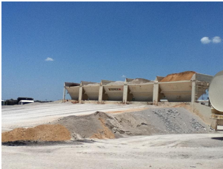
Figure 3.2 Aggregate Bins in Asphalt Plant in Bridgeport, TX
