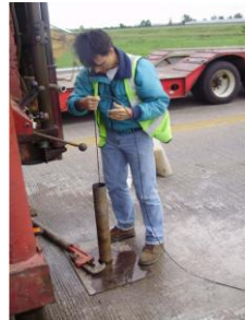
Figure 4.7 Sensor installation (courtesy of Bill Yu)
