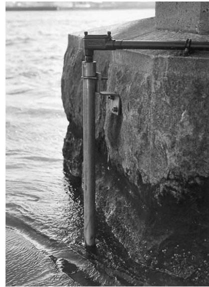
Figure 2.5. Detail of conduit to underwater sonar monitor (Copyright: Raimondo di Egidio 2002, cited by Hunter 2009).
