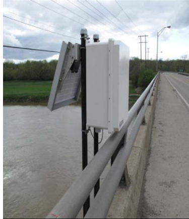
Figure5.4 Data acquisition box
