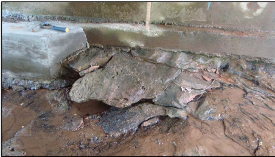
Figure 8 – Example of scalloped surface characteristic of abrasion scour (Coon Creek Bridge) .
