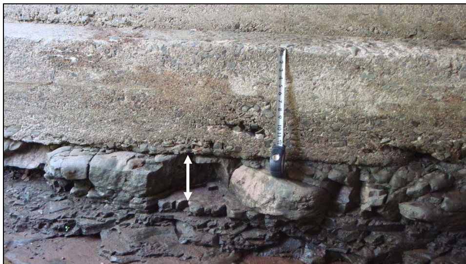
Figure 12 – Quarrying of jointed and bedded sandstone at Roaring Creek bridge site. Depth of scour (white arrow) measured as vertical thickness of block removed at base of pier.
