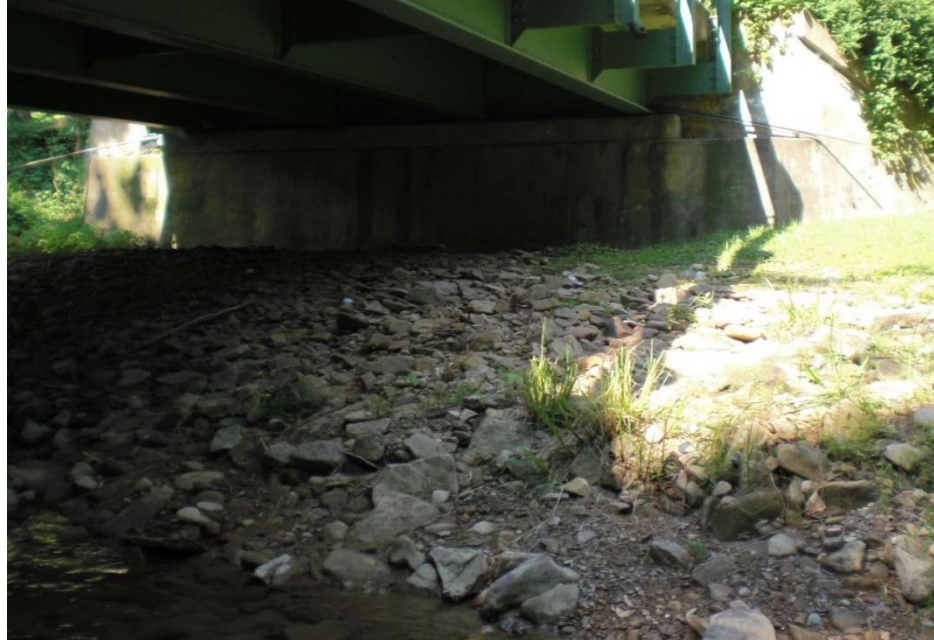
Figure 1- Photograph of abutment at Grassy Run project site. Water levels must rise before stream power begins to accumulate on the rocks under the abutment.
