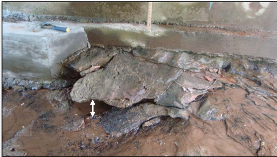
Figure 11 – Abrasion of highly weathered sandstone at Coon Creek bridge site. Note scalloped appearance of sandstone surface. Depth of scour, here as undercutting of protruding sandstone ledge, is indicated by arrow.
