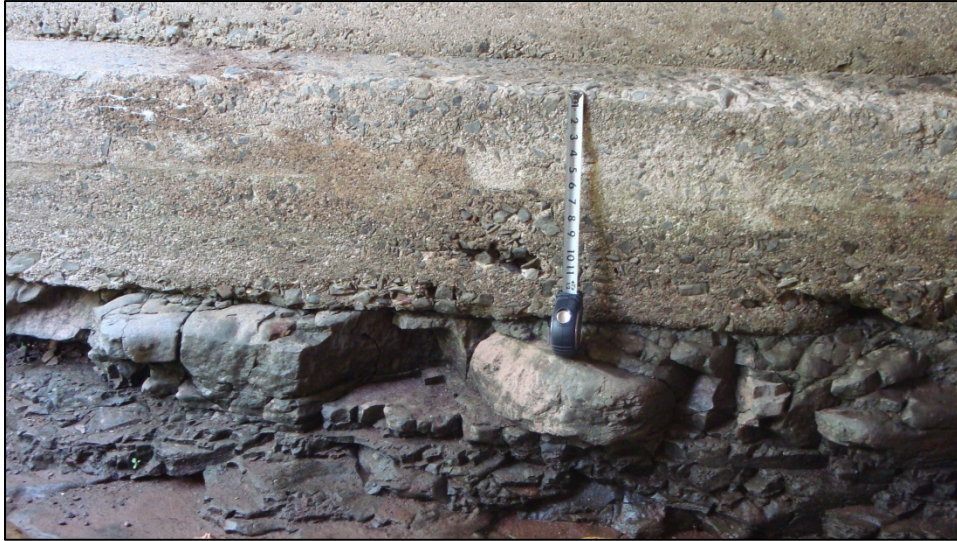
Figure 9 – Example of blocky appearance characteristic of scour by quarrying (Roaring Creek Bridge).
