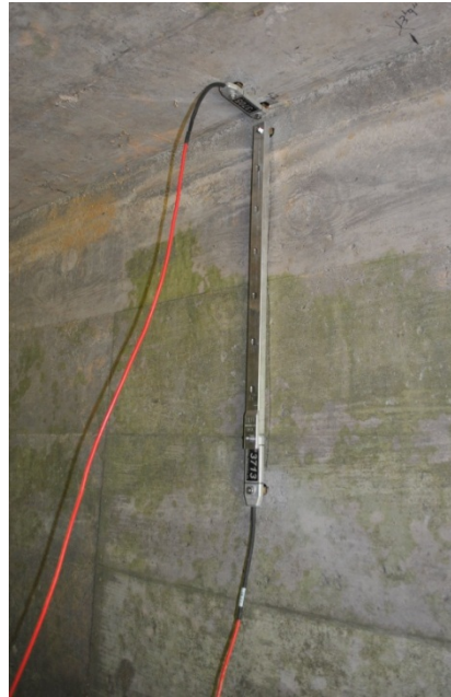
Figure 3-1– Two strain transducers, one installed without an extension rod on the culvert ceiling, and one installed with an extension rod on the culvert wall.
