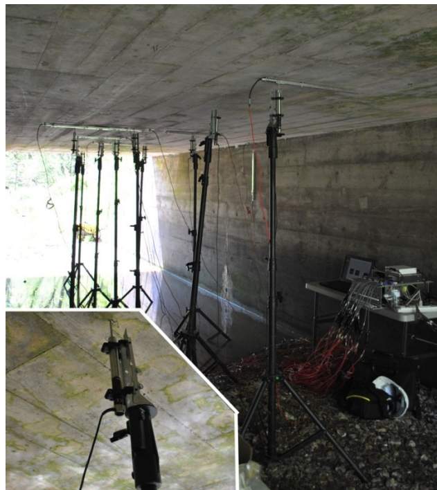
Figure 3-2 – LVDT tripods, with a closeup view of the LVDT mount shown in the inset. Data acquisition system can be seen at right.
