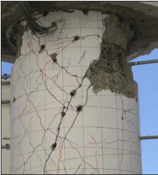
Damage state of as-built specimen SP2
