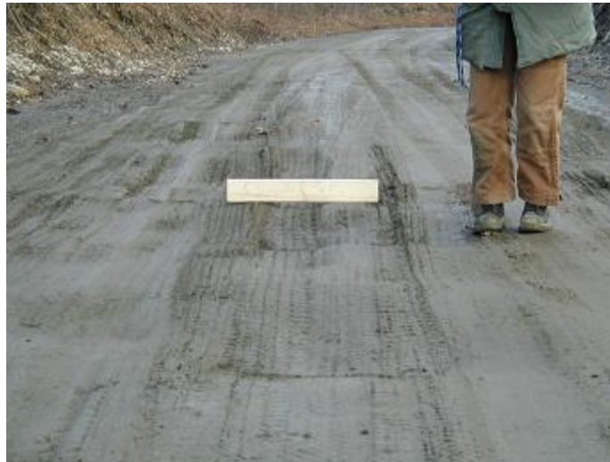
Figure 28. Rutting during spring-thaw (Henry et al. 2005)
