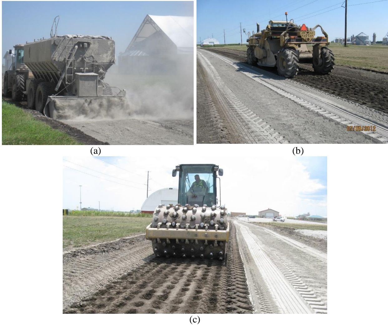
Figure 13. Photos showing typical chemical stabilization process: (a) spreading of cement stabilizer on subgrade, (b) mixing cement with subgrade material using a pulverizer, and (c) compaction of the soil-cement mixture using a padfoot roller (pictures from Boone County Expo Site, June 2012)
