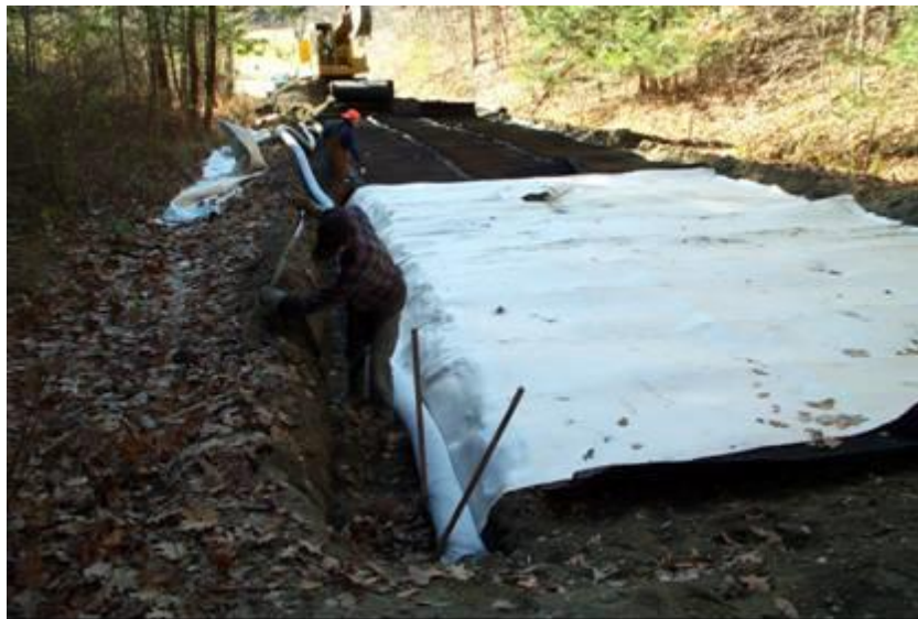
Figure 21. Geosynthetic capillary barrier drain (GCBD) installed on a test section over the subgrade/base interface in Vermont (Henry et al. 2005)
