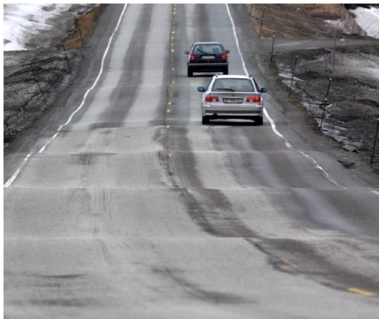
Figure 3. Frost-heave pavement damage in Norway (Ystenes 2011)
