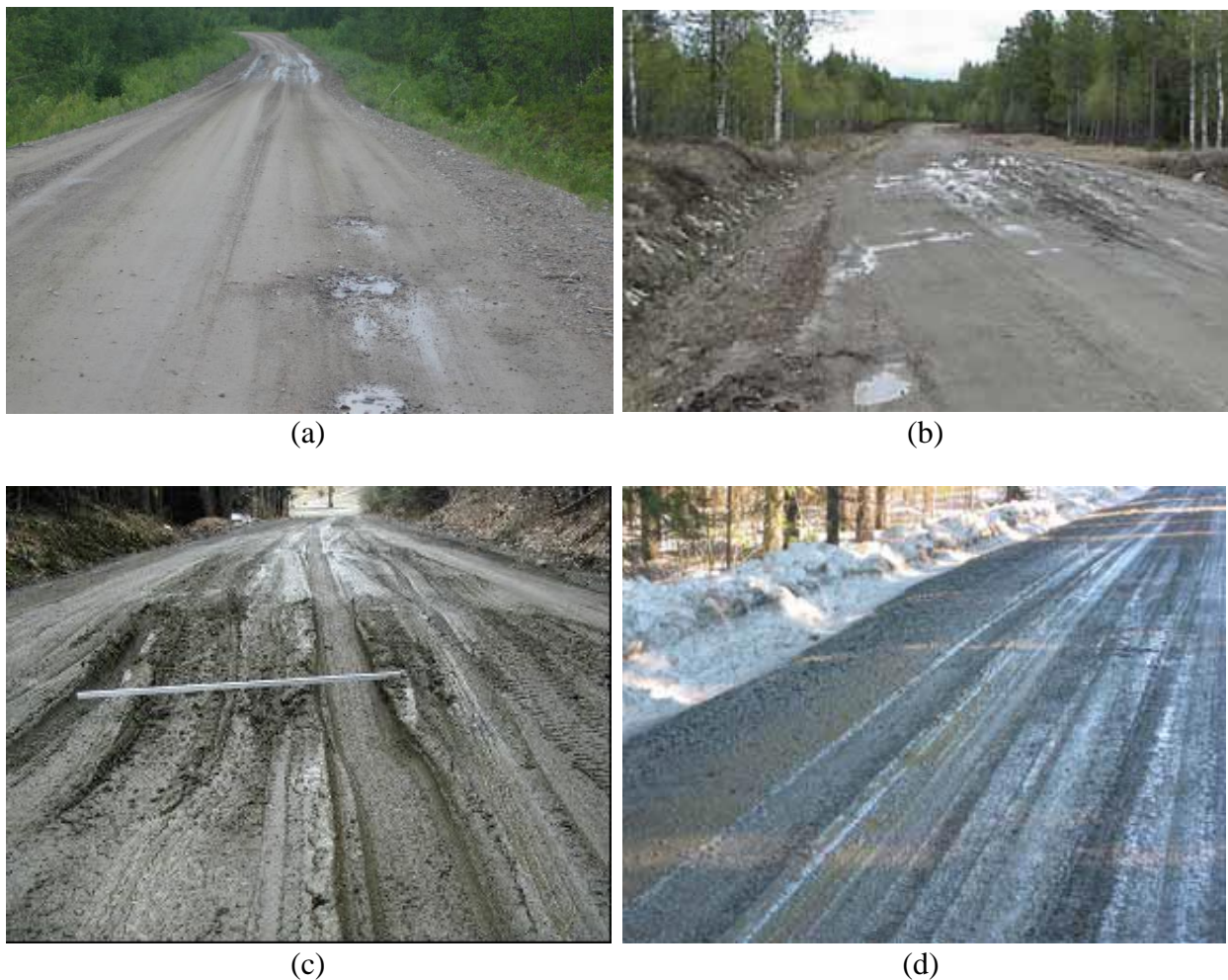
Figure 2. Freeze thaw damage on unpaved roadways: (a) potholes during July 2010 thawing season on a gravel road near Boden, Sweden (Christoffersson and Johansson 2011), (b) structural spring thaw damage on a moraine soil in Kemijarvi, Finland (Saarenketo and Aho 2005), (c) rutting damage on a gravel road in Vermont shortly after adding 6 in. of gravel to saturated subgrade in April 2002 (Henry et al. 2005), (d) early phase of surface thaw-weakening on a gravel road in Finland (Saarenketo and Aho (2005))
