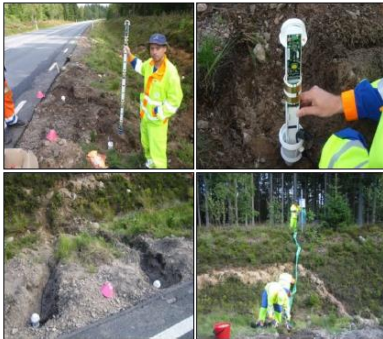
Figure 35. Moisture probes with wireless data transfer installation at a ROADEX project site in Southern Sweden (Saarenketo and Aho 2005)
