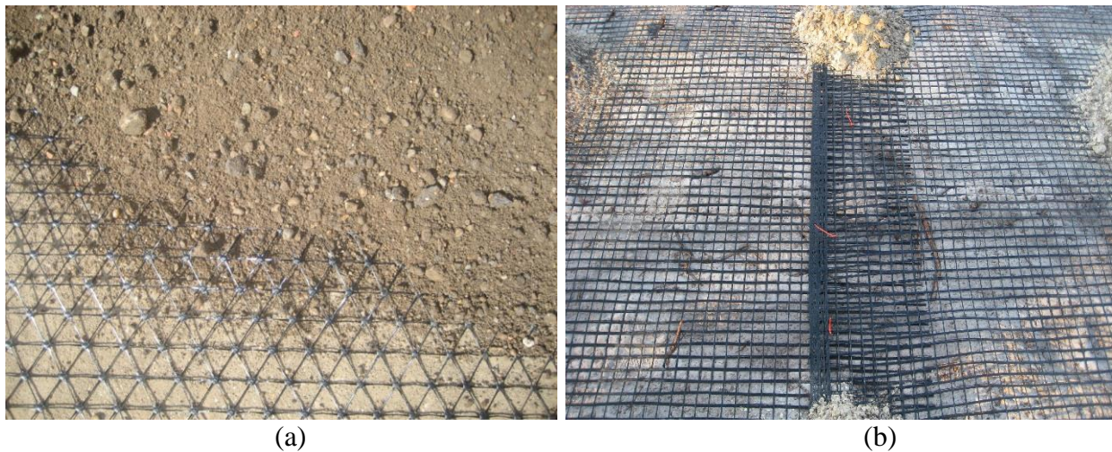
Figure 20. Polymer geogrids placed at subgrade/aggregate layer interface: (a) triaxial geogrid, and (b) bi axial geogrid (pictures from Boone County Expo Site, June 2012)
