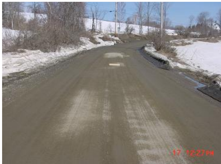
Figure 14. Cement stabilized section during thawing period from a test site in Vermont (picture from March 17, 2003, Henry et al. 2005)
