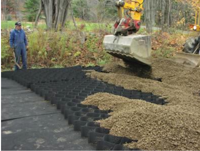
Figure 22. Geocells placed over non-woven geotextile on a test section in Vermont (Henry et al. 2005)
