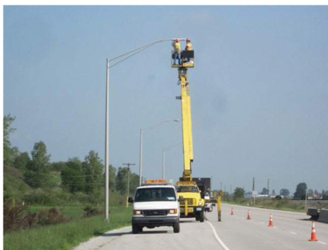
Figure 4.6 Field luminaire installation.
