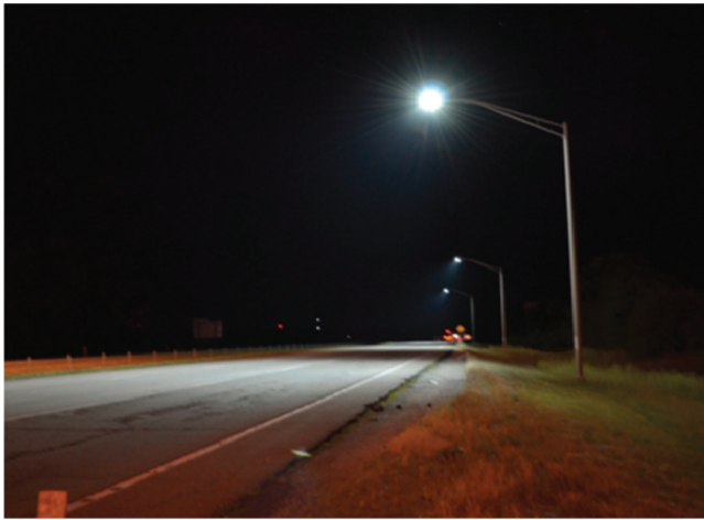
Figure 2.4 Plasma lighting installed in test zone.
