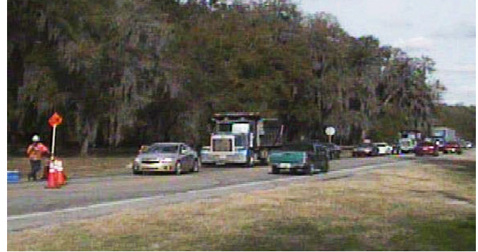
Work zones on Florida's many two-lane roads must be carefully designed to minimize impacts on drivers.
