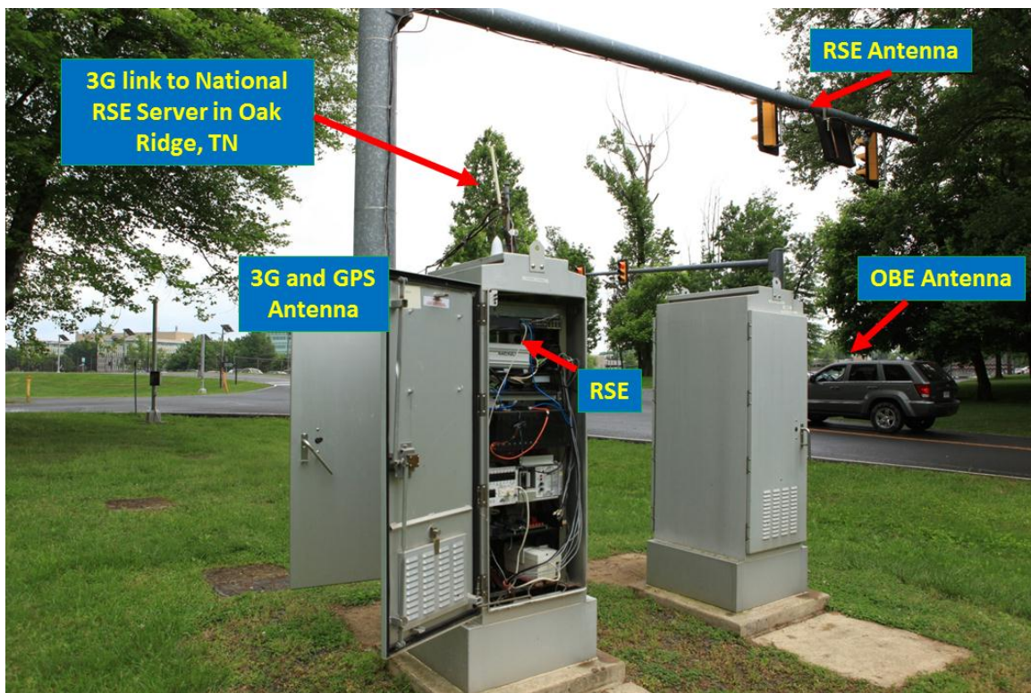
Figure 5-6. TFHRC's Cooperative Vehicle Highway Test Bed (CVHT) Intelligent Intersection (Source: Turner-Fairbank Highway Research Center, FHWA)
