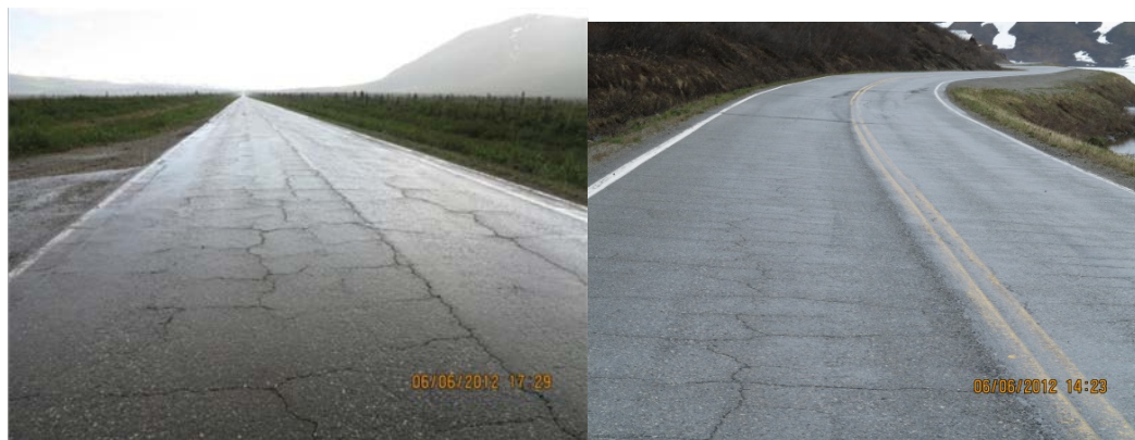
Figure III.9 Lessor thermal cracks—severe (no sealant)
