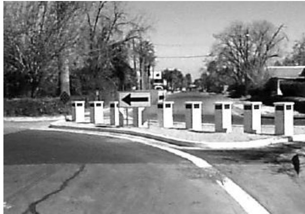
Figure 2-14: Traffic Diverter (Harkey and Zegeer, 2004)
