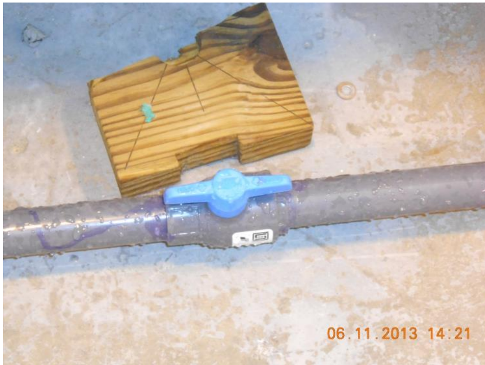
Figure A-32. Water chiller overflow valve in the "open" position
