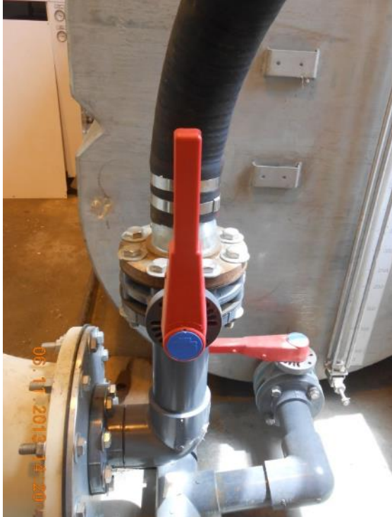
Figure A-27. Downstream butterfly valve in open position
