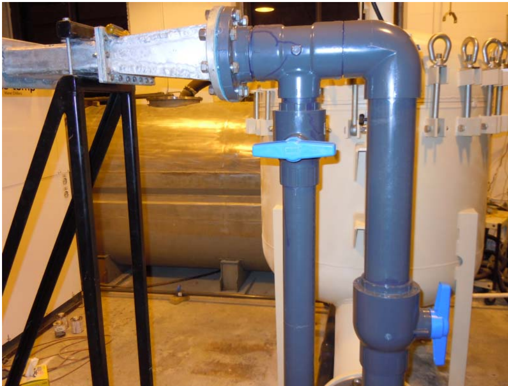
Figure A-18. SERF downstream valve system
