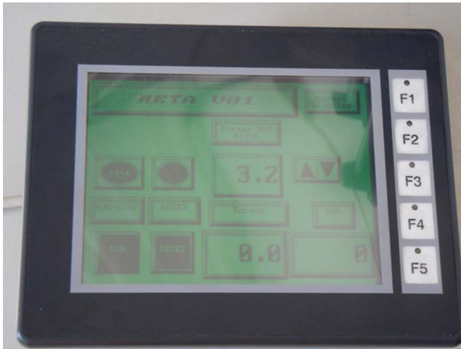
Figure 2-11. RETA control screen
