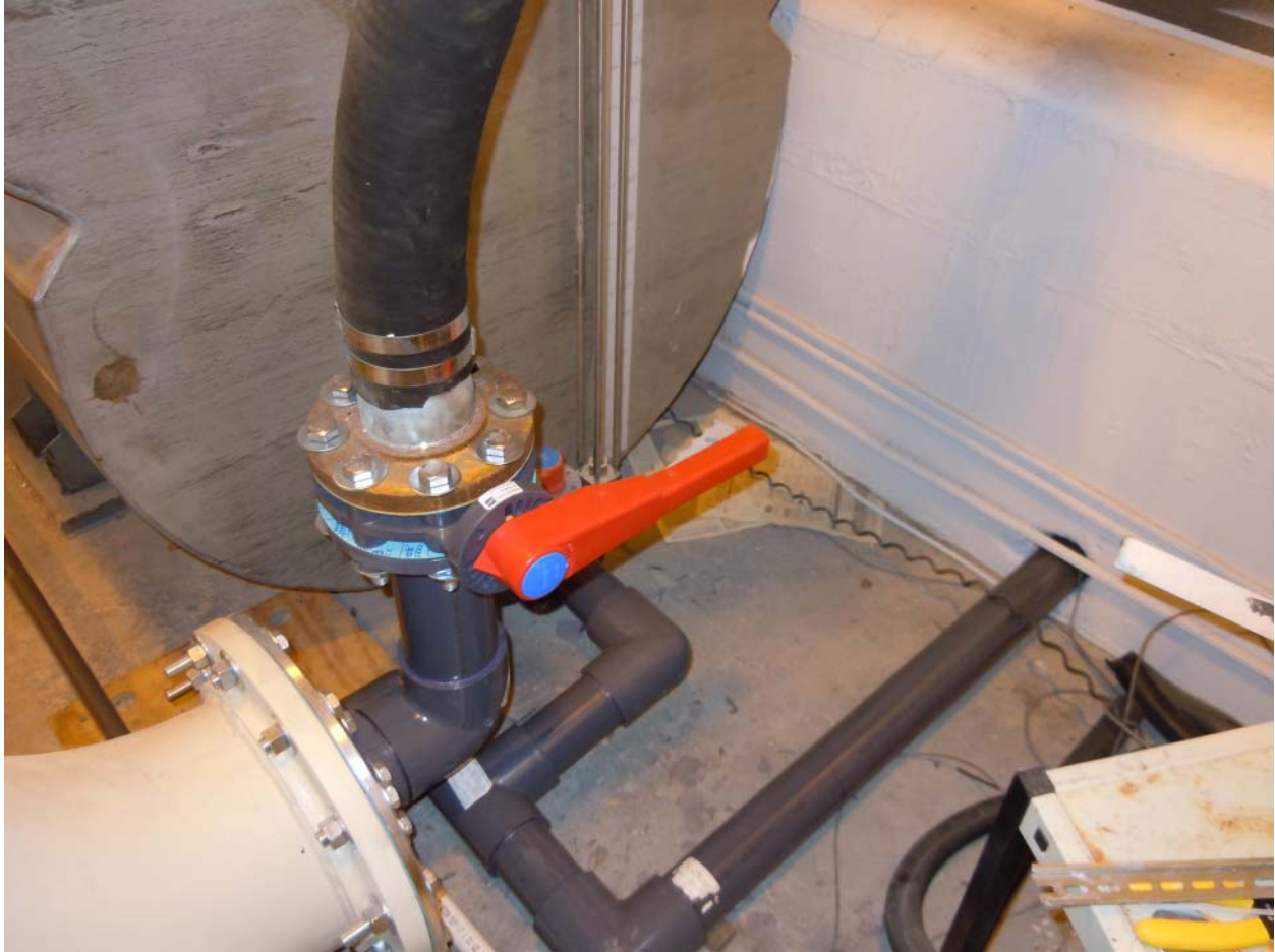
Figure A-19. Downstream pump butterfly valve
