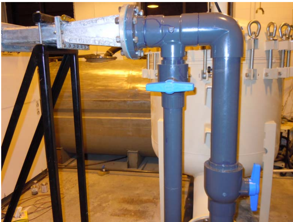
Figure A-26. Downstream flow valve and drain valve in open and closed positions, respectively
