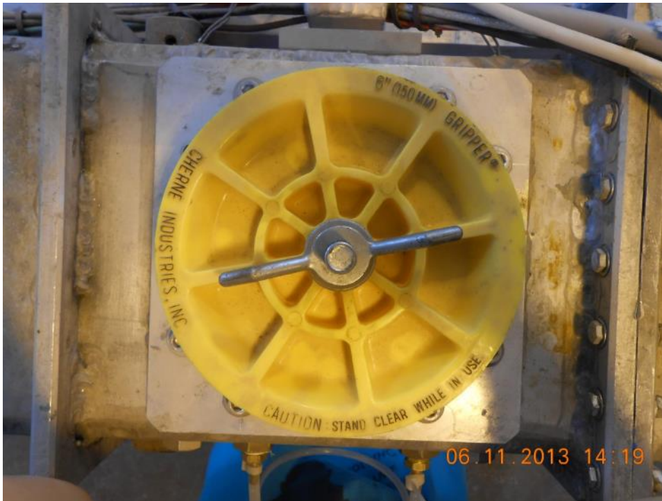
Figure A-23. Shear stress sensor top hatch PVC plug
