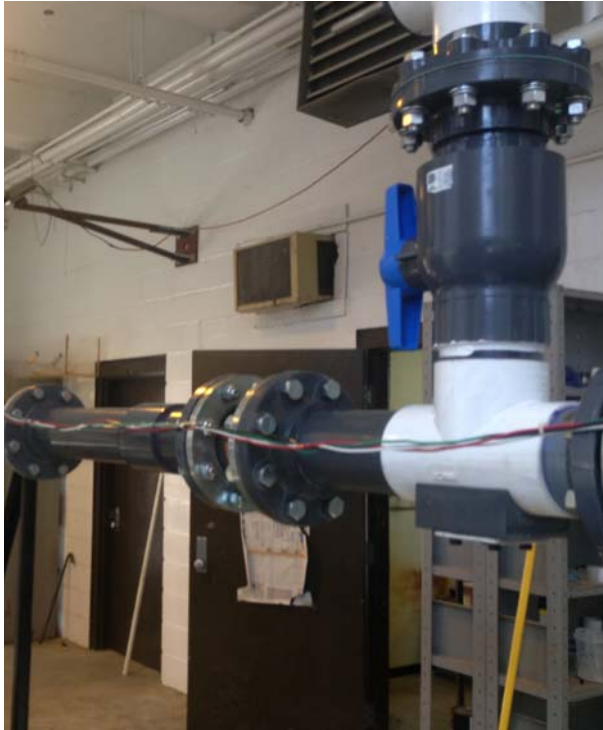
Figure A-15. Sand injector shut-off valve
