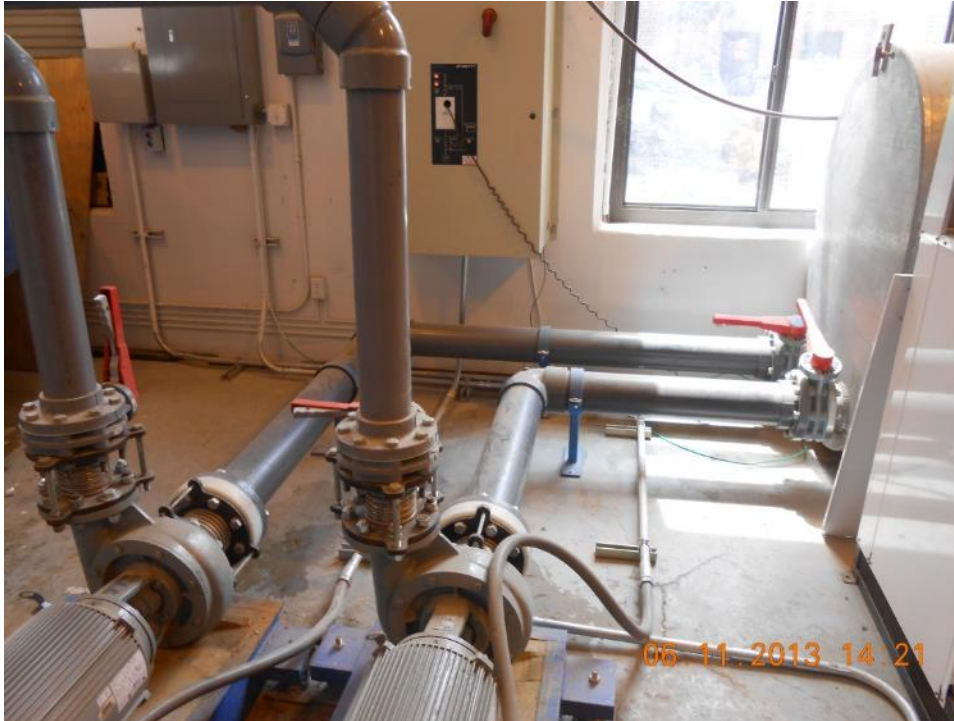
Figure A-25. Upstream butterfly valves in the “open” position showing configuration when one pump is used
