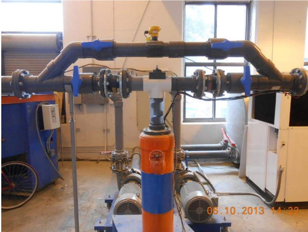
Figure 8-2. Photograph of original sand injector installed in SERF with valve system
