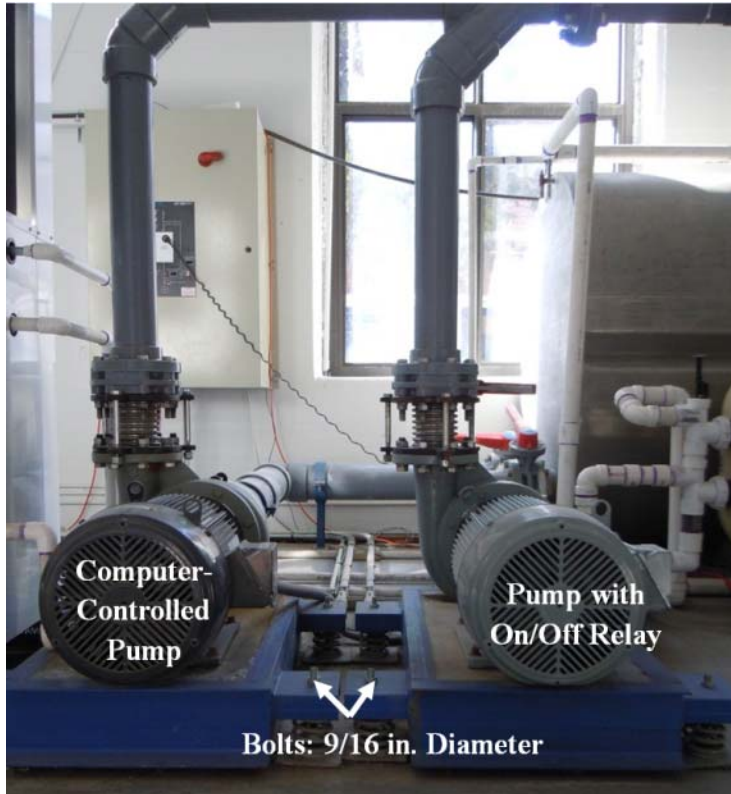
Figure 2-3. Photograph of SERF pumps
