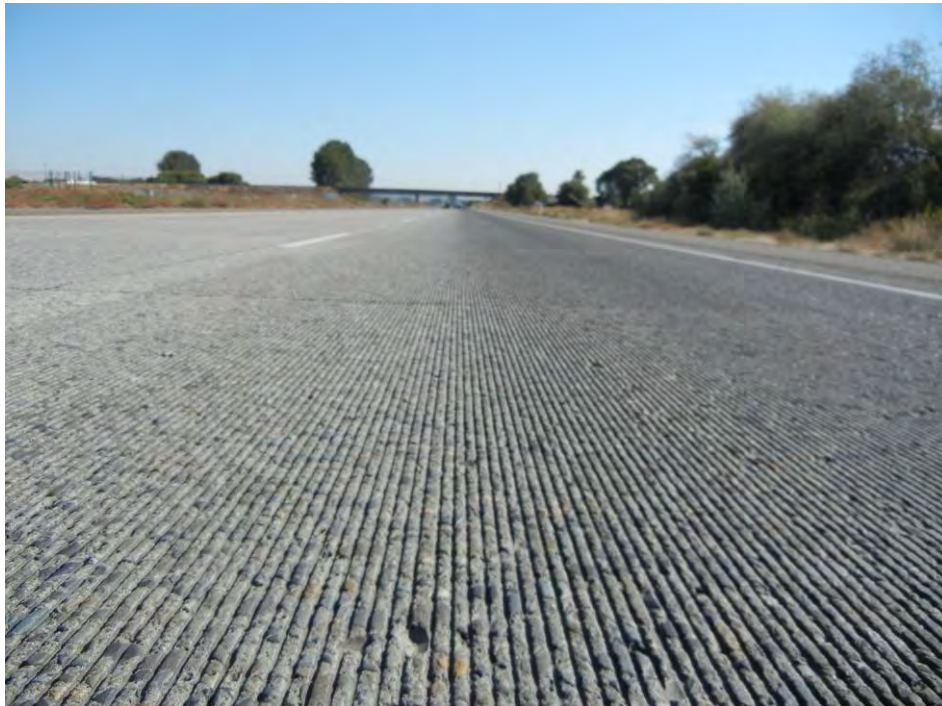
Figure 17. Another view of the attrition on the NGCS, note missing aggregate, October 2013.
