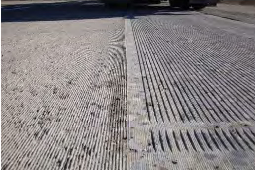
Figure 11. Conventional diamond ground surface on the left, first pass of NGCS in the middle and final pass of the NGCS on the right.
