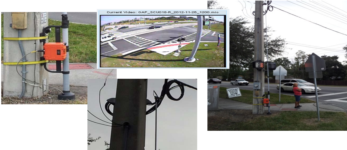
Figure 3-2: VCU Attached to an Electric Pole with Camera at 20 Feet High
