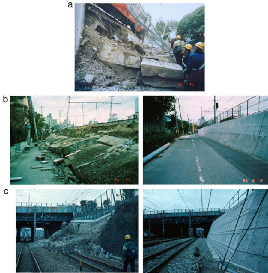
Figure 2-1: Typical forms of damage to (a) gravity (b) gravity leaning and (c) masonry unreinforced walls in the 1995 Kobe earthquake [5]
