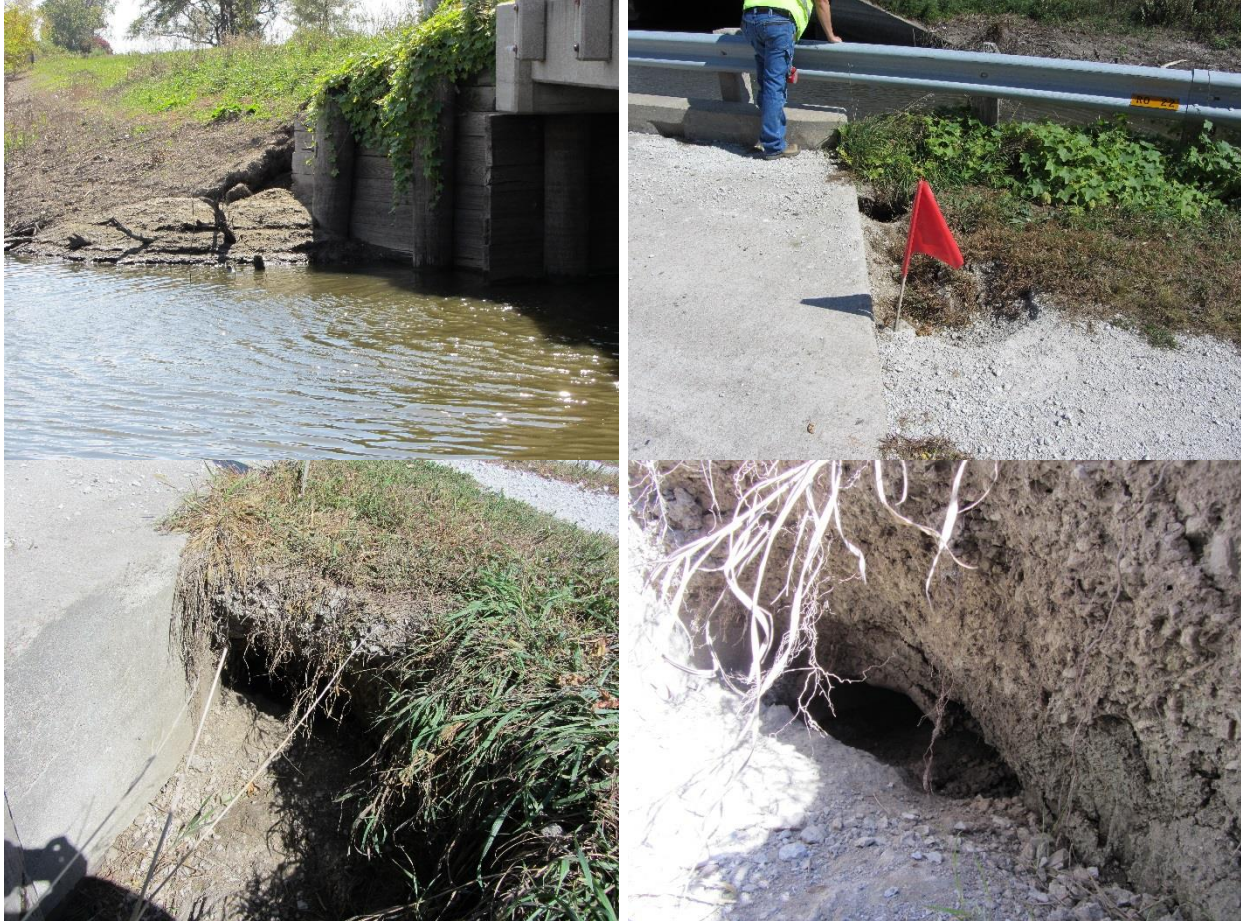
Figure 44. Scouring and erosion of bridge backfill material around a timber abutment supporting a concrete bridge deck – Pottawatamie County (Photos taken on 9/21/11)
