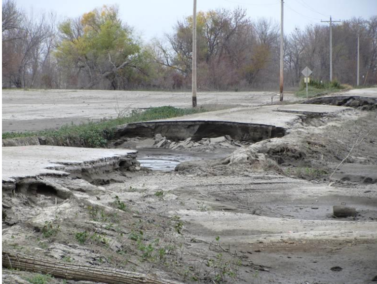
Figure 52. Gravel road segments washed away during floods – Fremont County (Photo taken on 10/26/11)
