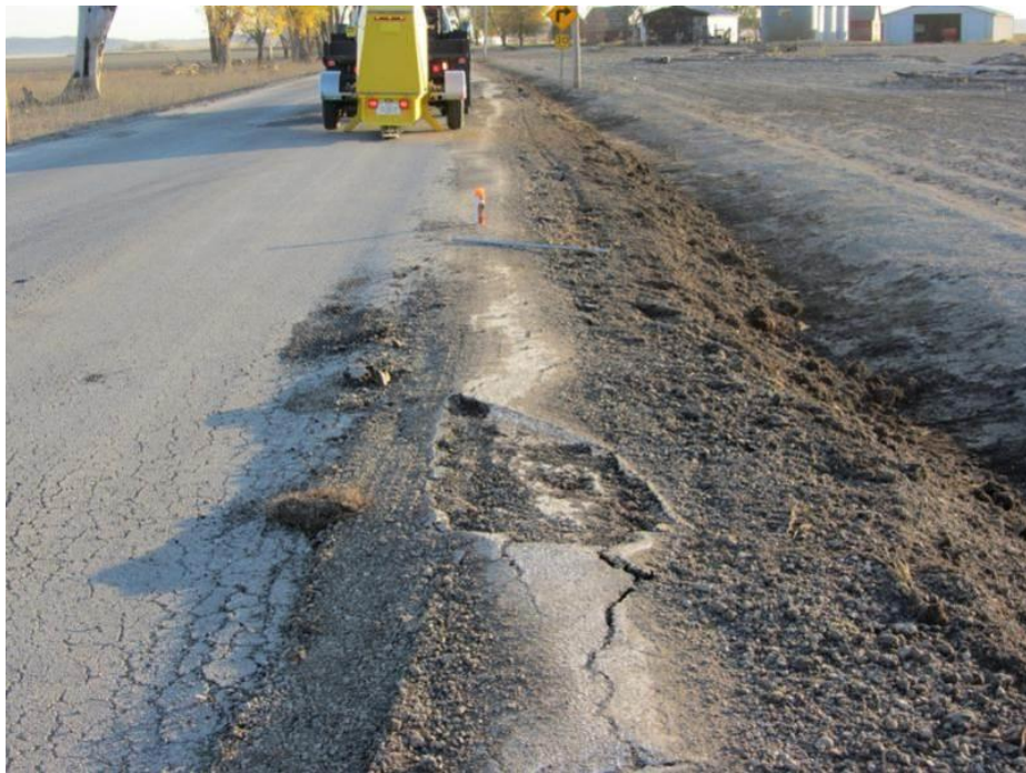
Figure 162. Rutting observed on the surface and washed out shoulders during flooding on TS4 – Fremont County (Picture taken 10/28/11)
