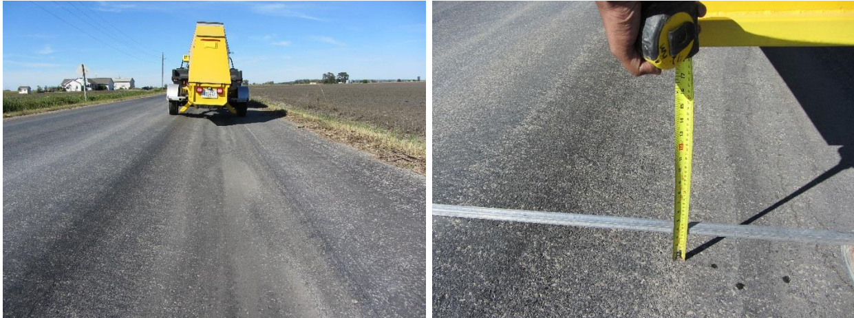
Figure 82. Rutting observed near the east end of the test segment (near test location D-38) (photo taken on 9/23/11) on TS4 – Pottawattamie County
