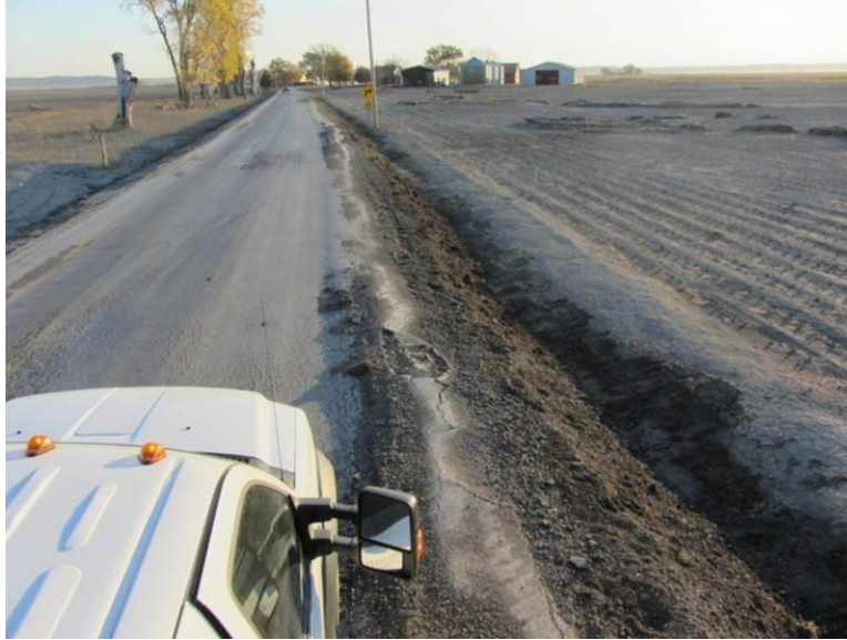
Figure 48. Rutting along right wheel path on chipseal surfaced gravel road and erosion of granular shoulder during flooding – 220th Street, Fremont County (Photo taken 10/26/11)
