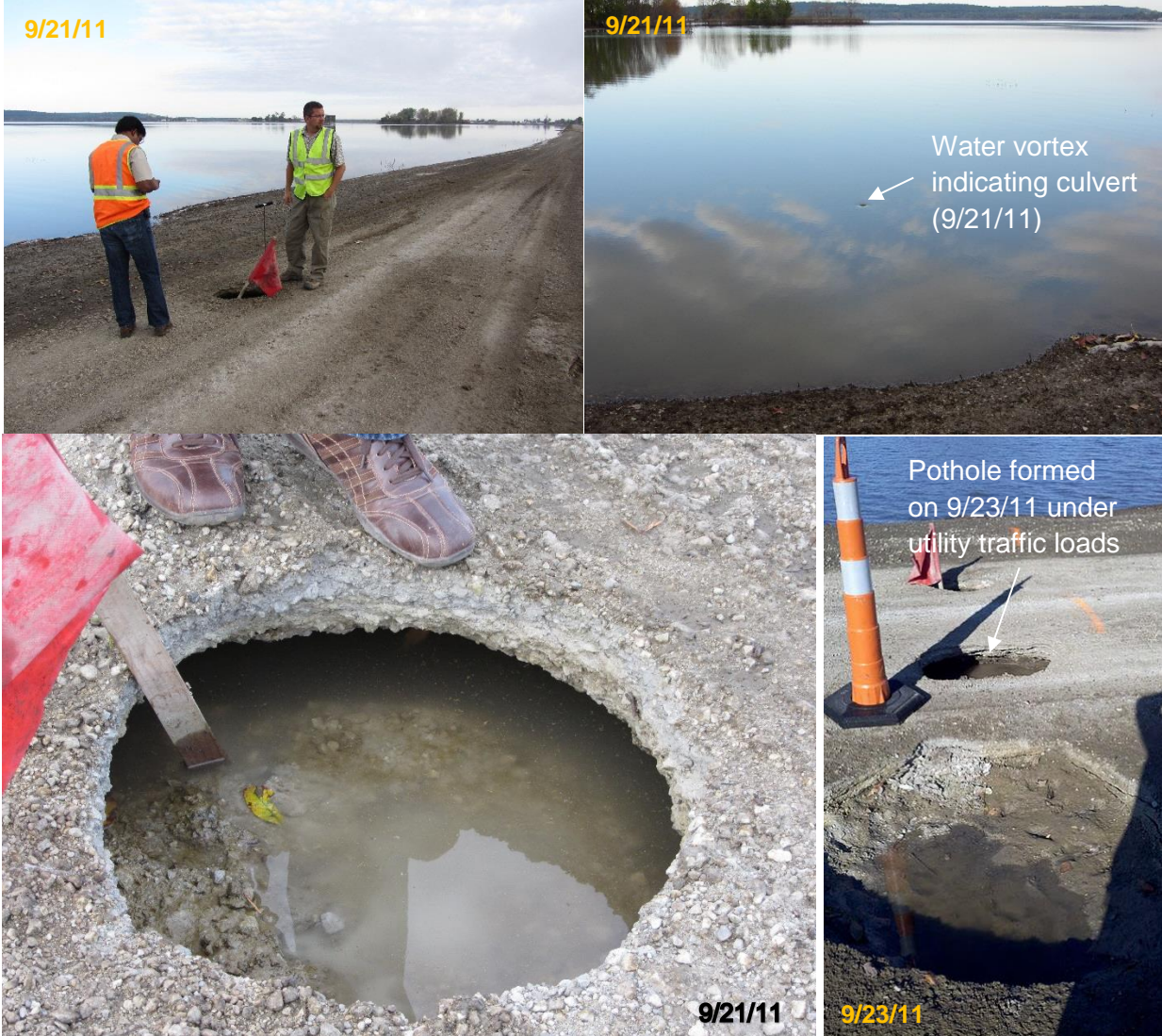
Figure 89. Potholes (with about 0.5 m (1.5 ft) diameter) under gravel road due to erosion of backfill material around a culvert located beneath the road TS 5 (Photos taken on 9/21/11 and 9/23/11) – Pottawatamie County
