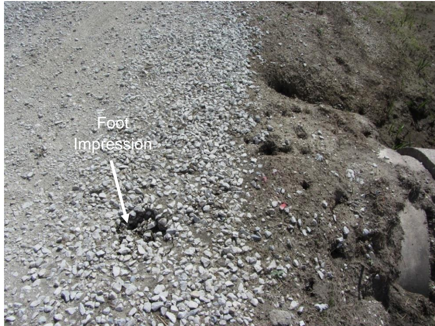
Figure 92. Loose backfill material around culvert replaced after flood waters receded on TS5 (Photo taken on 4/5/12) – Pottawattamie County
