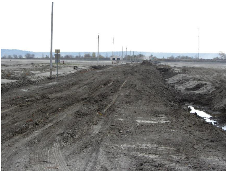
Figure 53. Reconstruction of a gravel road washed away during floods and deposited with silt and sand– Fremont County (Photo taken on 10/26/11)
