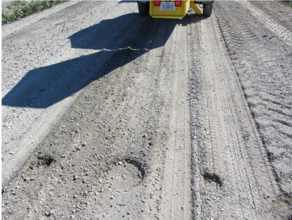
Figure 110. FWD plate depression and rutting under truck wheels near culvert (Picture taken on 9/23/2011) – Pottawattamie County
