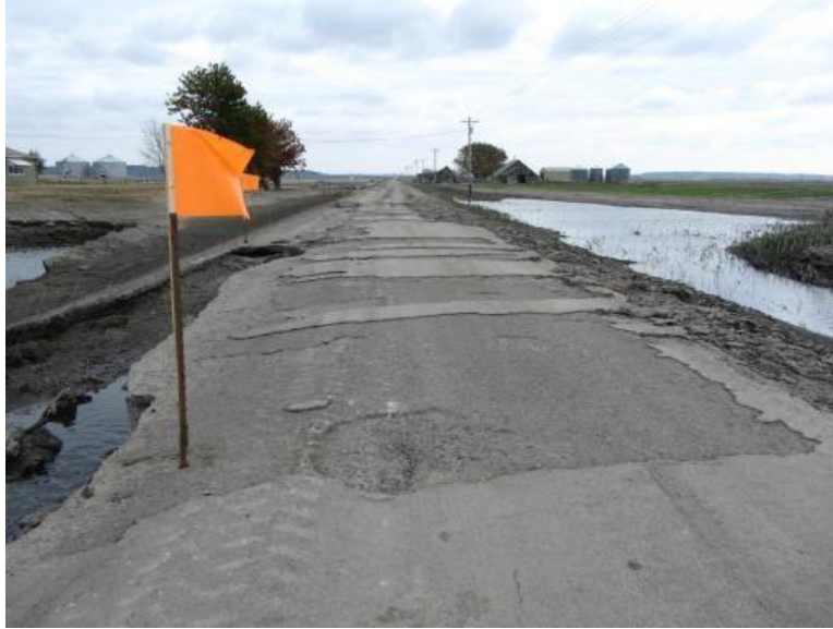
Figure 50. Delaminated or stripped chipseal surfacing – Fremont County (Photo taken on 10/26/11)
