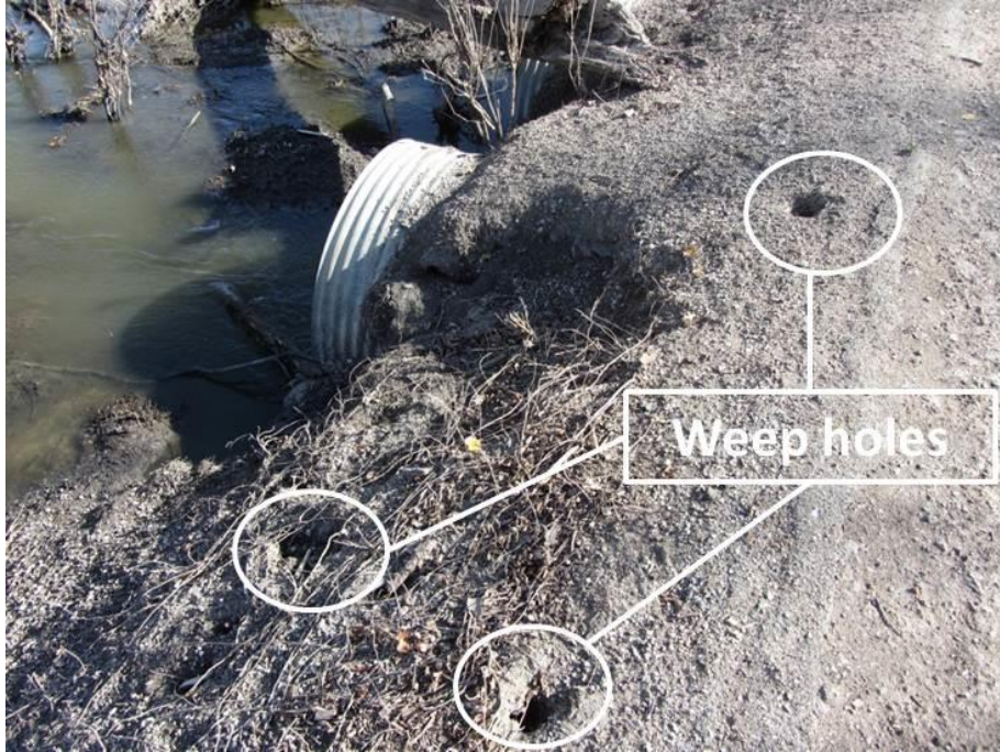
Figure 122. Weep holes around culvert inlets on TS7 (Picture taken on 10/25/11) – Pottawattamie County
