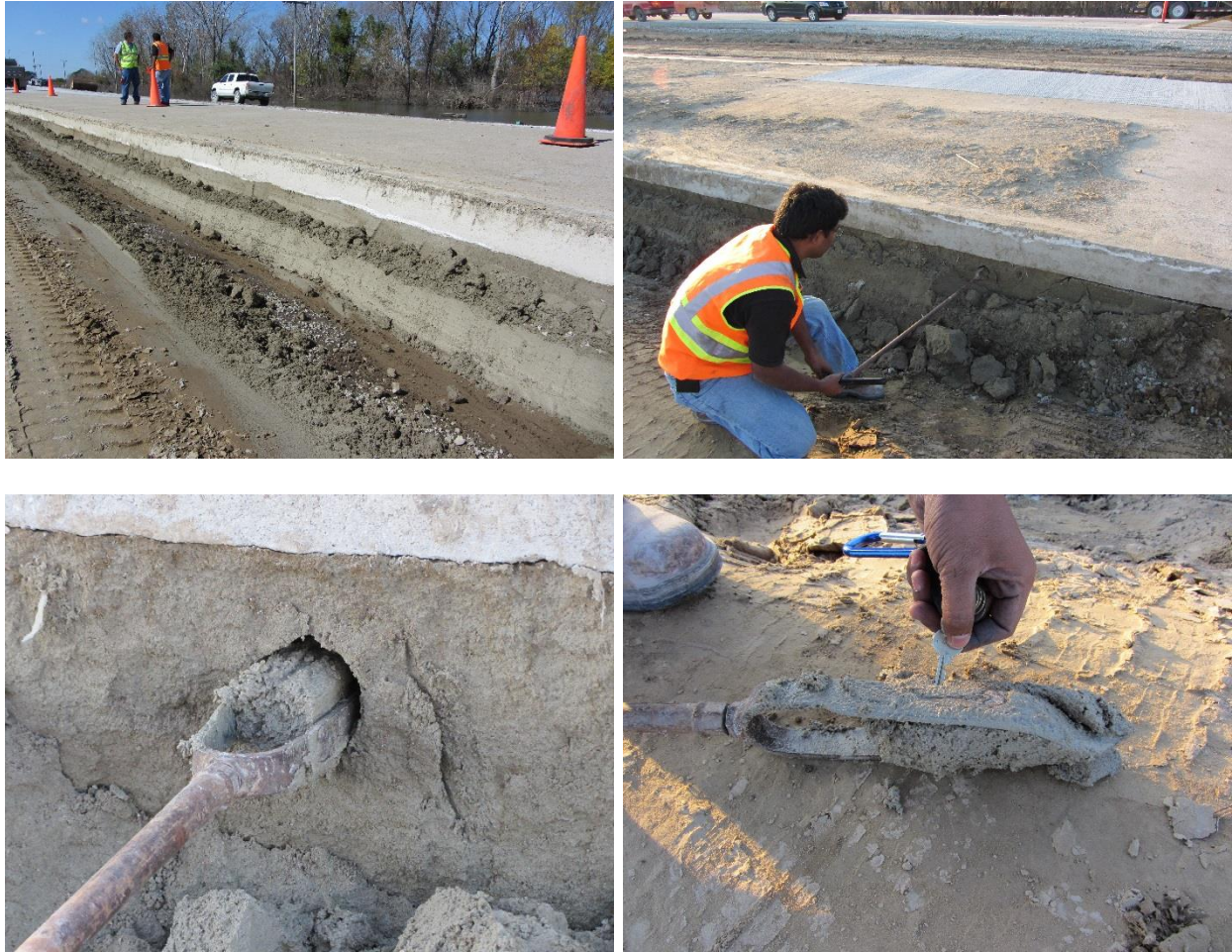
Figure 63. Eroded base material and voids under PCC pavement filled with cement grout – TS2 [Note: Cement grout was placed two days prior to taking these photos] (Photos taken on 9/21/11) – Pottawattamie County
