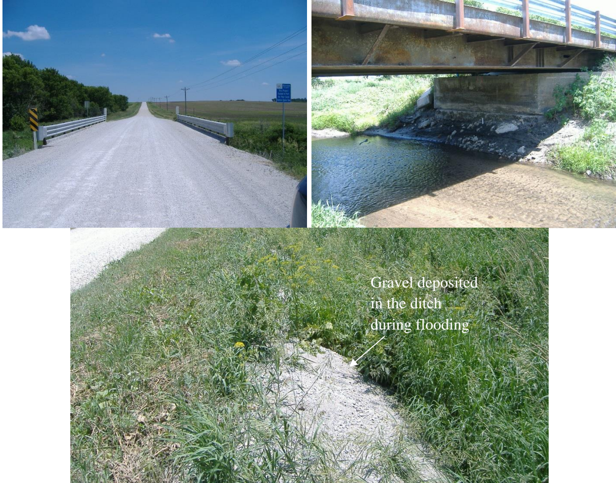
Figure D42. Pictures of a bridge site in Buchanan County (250 th Street) after flash flooding occurred in May 2013
