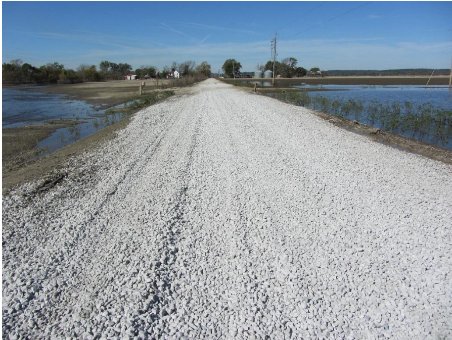
Figure 113. Location of newly placed gravel on TS6 over a metal pipe culvert (Picture taken on 9/23/11) – Pottawattamie County
