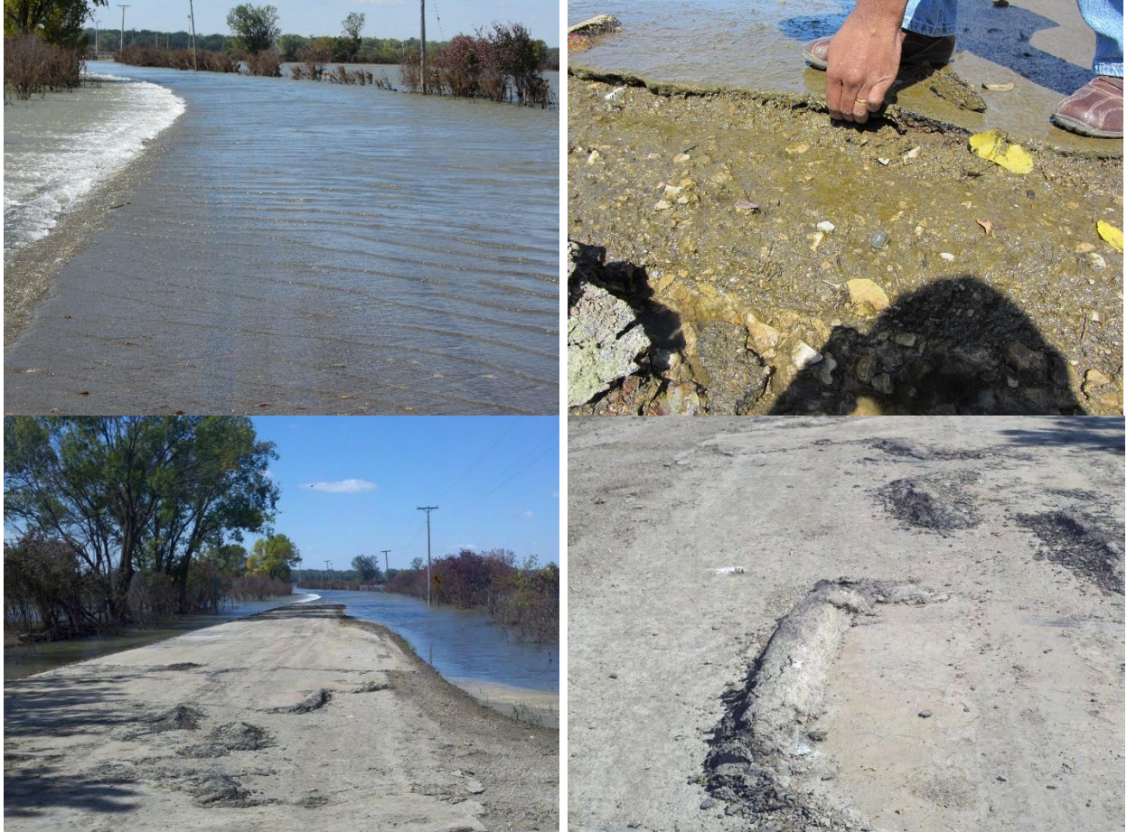
Figure 42. Water overtopping a thin chipseal coat surfaced road underlain by oil stabilized granular base on 9/21/11 showing delamination of chipseal and rolled asphalt at the surface – Desoto Avenue, Pottawattamie County (Photos taken on 9/21/11)
