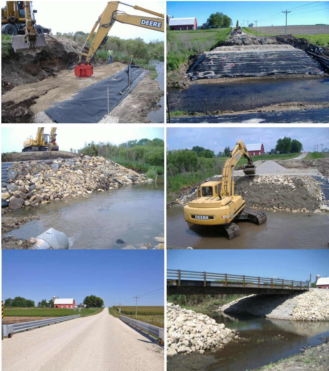
Figure D39. Pictures of a bridge site in Buchanan County (Olympic Ave.) during construction of GRS fill in bridge abutments, placement of riprap and grout cover for erosion protection, and the finished bridge in 2011 (Vennapusa et al. 2012)
