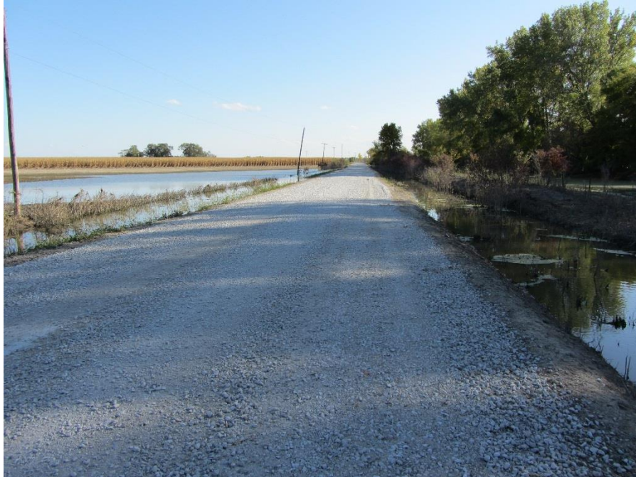
Figure 72. New gravel placed at the middle of the segment following flooding on TS3 (Photo taken on 9/21/2011) – Pottawattamie County
