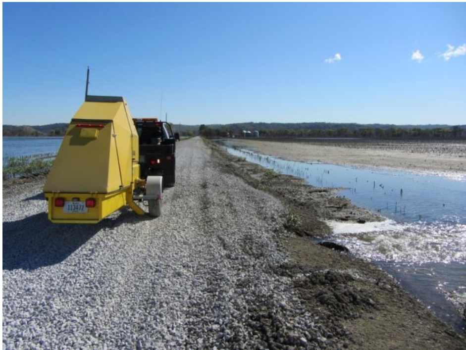
Figure 111. Newly placed gravel showing rutting near culvert (Picture taken on 9/23/2011) – Pottawattamie County
