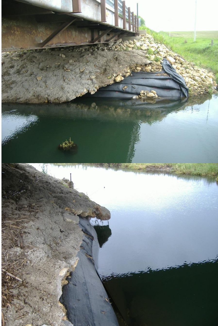
Figure D41. Pictures of a bridge site in Buchanan County (Olympic Ave.) after flash flooding occurred in May 2013
