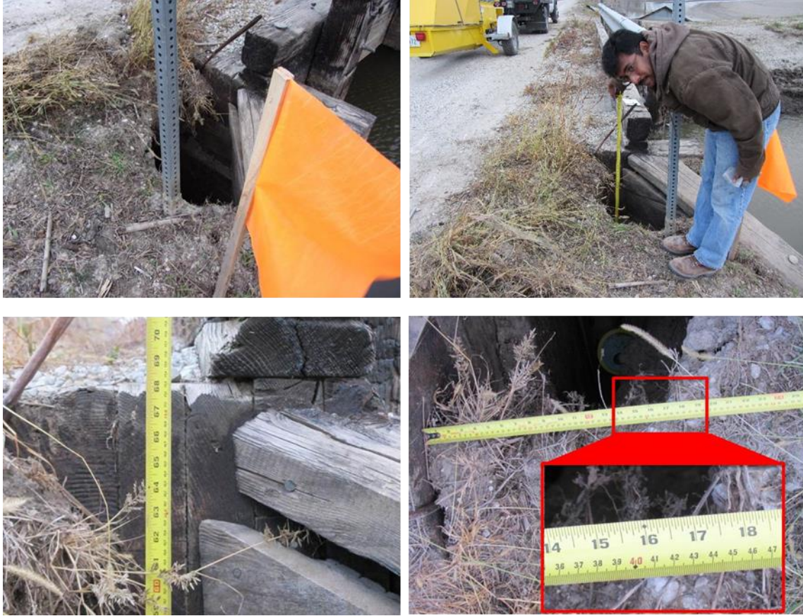
Figure 146. Void behind the west abutment wall due to erosion of backfill material at TS2 bridge (Pictures taken on 10/26/11) – Fremont County
