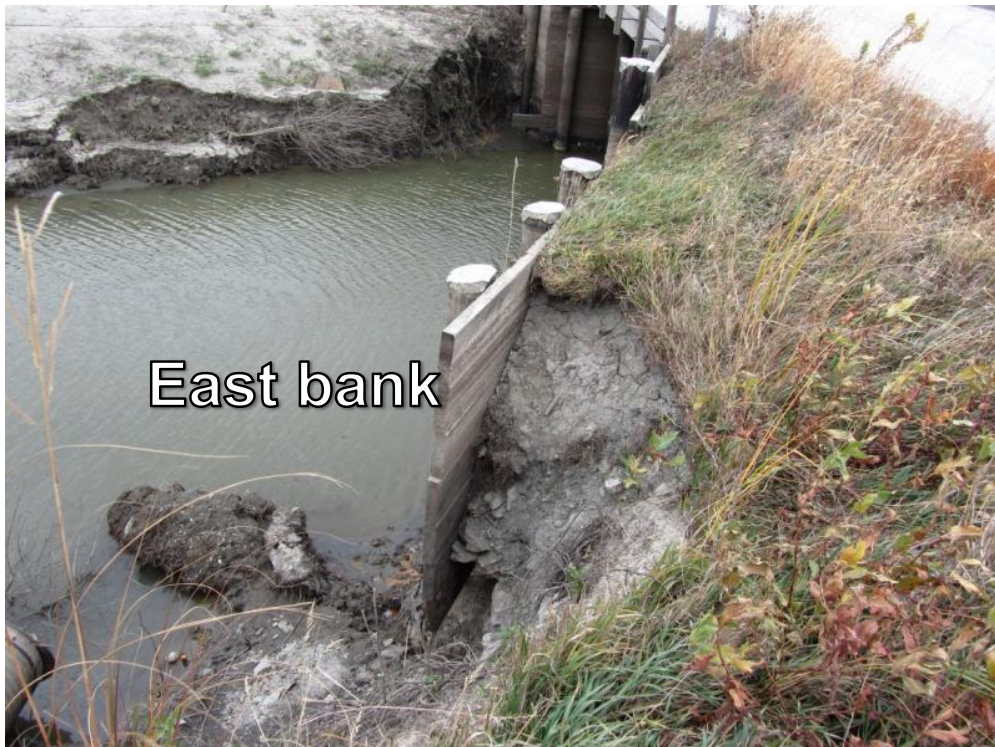
Figure 133. Erosion of backfill material behind the wing wall on TS1 (Picture taken on 10/26/11) – Fremont County
