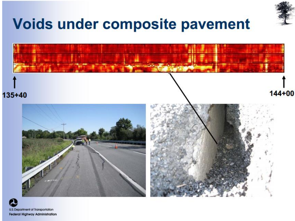
Figure D17. GPR scan map showing voids under composite pavement (Yu 2012)
