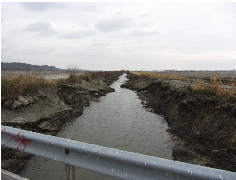
Figure 54. Erosion of backfill material around timber back wall supporting a timber bridge crossing a creek – Fremont County (Photos taken on 10/26/11)
