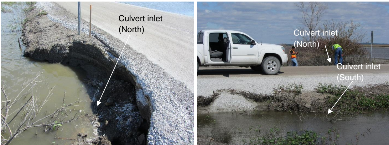
Figure 43. Clogged culvert inlets due to scouring and erosion of embankment material beneath chipseal coat surfaced road on 9/21/11 – Desoto Avenue, Pottawatamie County (Photos taken on 9/21/11)
