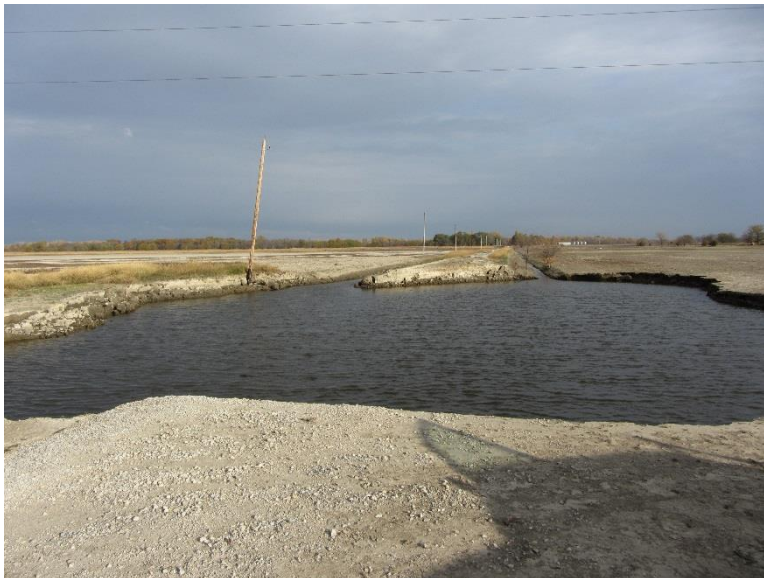
Figure 51. Full breach of a gravel road (about 100 m (330 ft) long) – Fremont County (Photo taken on 10/26/11)
