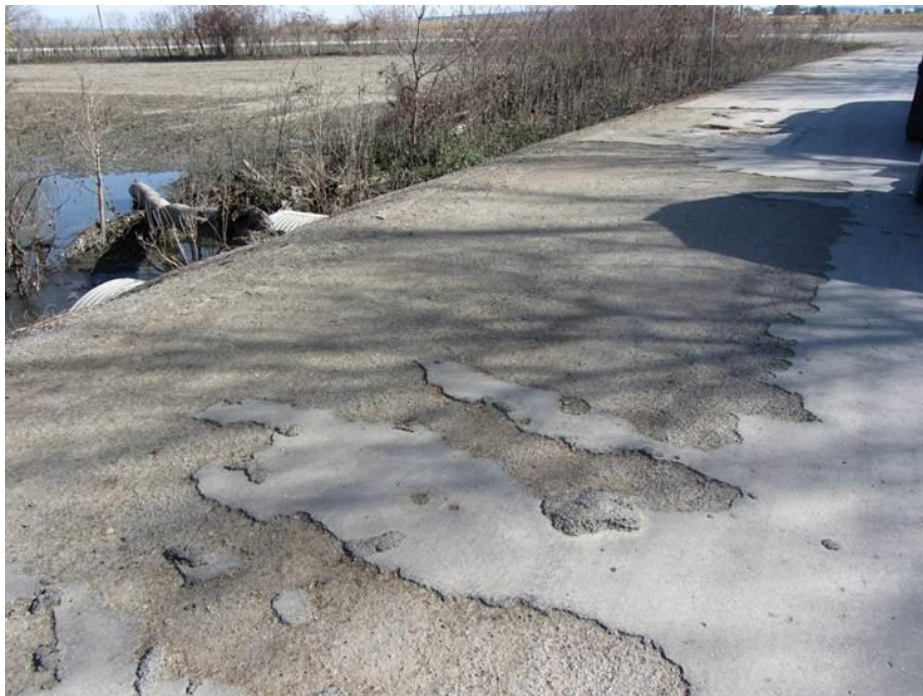
Figure 121. Delaminated surface chipseal on Desoto Avenue due to flood waters overtopping the roadway (Pictures taken on 10/25/11) – Pottawattamie County
