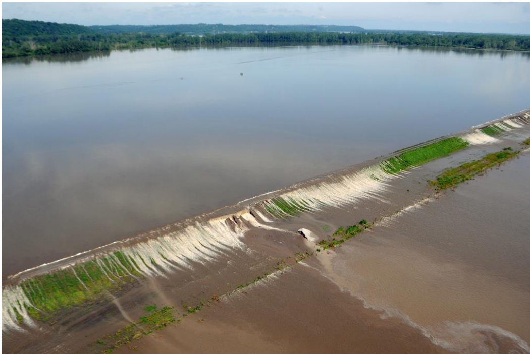
Figure 13. Aerial photo of the overtopping of Federal levee 550 near Highway 136 in Atchison County, Missouri, on June 19, 2011 (Image Courtesy of USACE http://www.flickr.com/photos/usacehq/5849817627/in/photostream/ )
