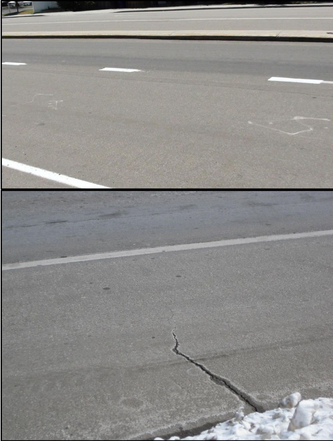
Figure 5.2 SR 111 on June 13, 2012, no visible thermal distress (Top) and January 23, 2013, showing a thermal crack (Bottom)
