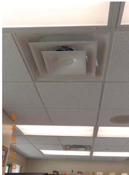
Figure 4.10. T8-fluorescent lamps are typically used in the office area
