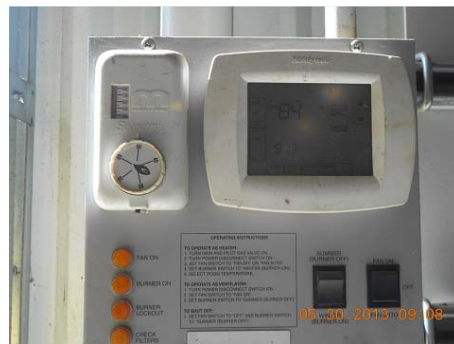
Figure 4.12. Control panel for make up air units.
