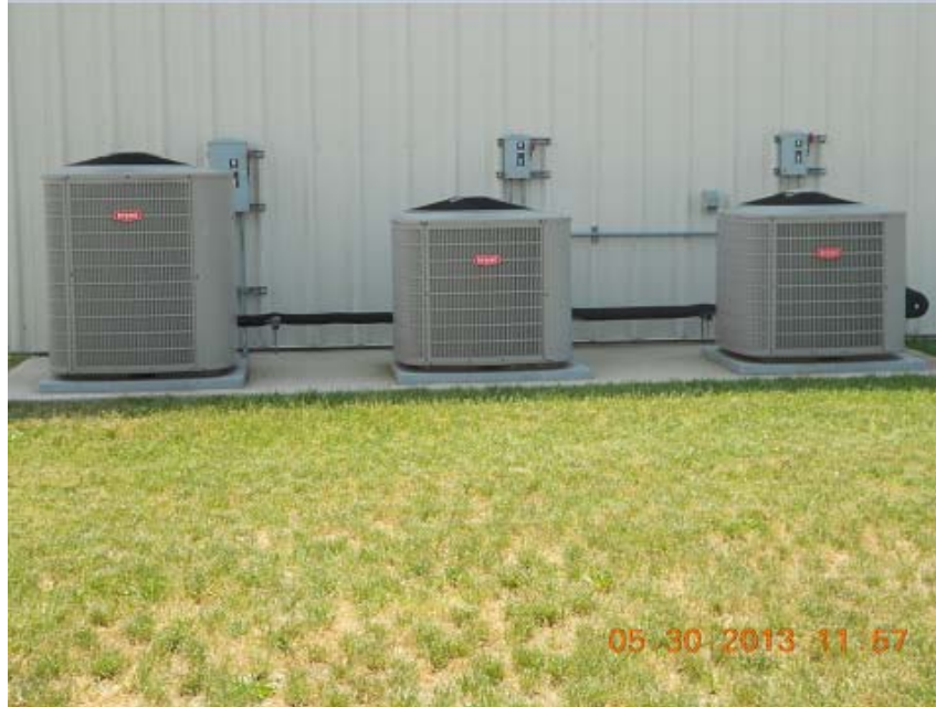
Figure 4.5. Outdoor electrical condensers provide space cooling for the office area
