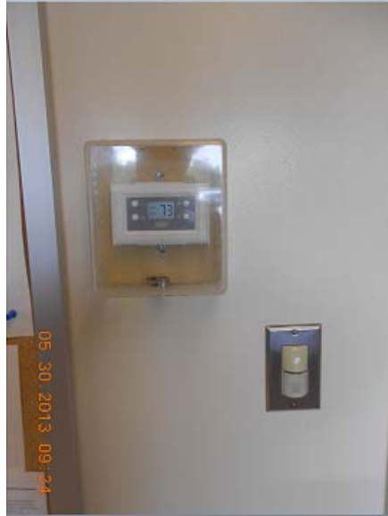
Figure 4.11. Thermostat controls and occupancy sensors are used in office area to control HVAC equipment and lighting respectively.
