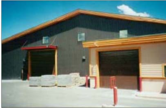
Figure 6.8. An SAH collector installed on a gable wall on the BigHorn Home Improvement Center in Silverthorne, Colorado. Photo credit solarwall. http://solarwall.com/media/download_gallery/BigHorn-SolarWall.pdf
