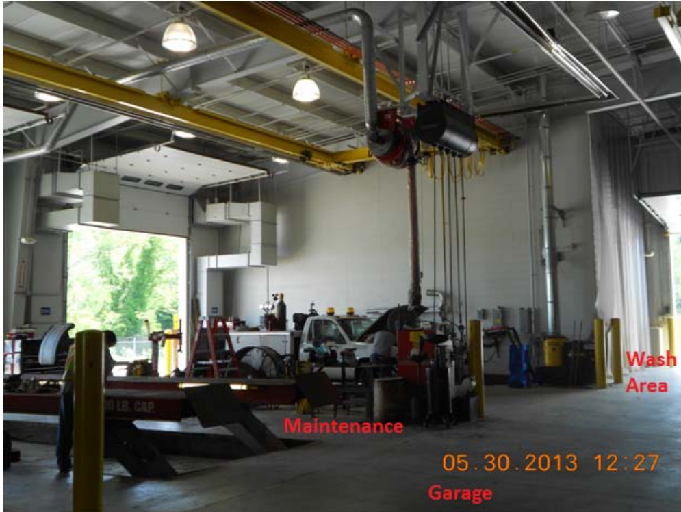
Figure 5.1. Several functional spaces with different heating requirements are combined in many existing ODOT facilities.
