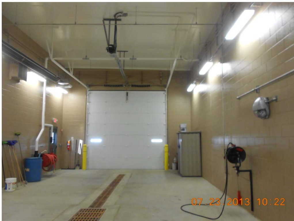
Figure 5.5. Truck washing building in New Lucas County garage is constructed of CMU instead of structural steel to reduce corrosion problems.
