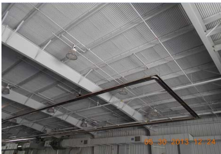
Figure 4.2. Radiant heaters provide space heating for the maintenance/garage area
