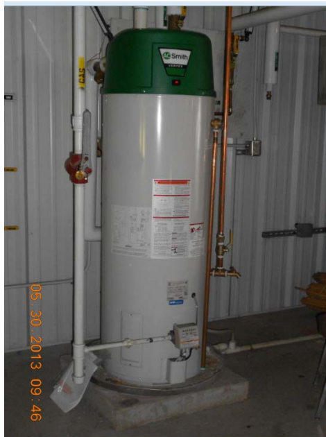
Figure 4.6. Water heating for sanitary uses is provided by a gas-fired water heater
