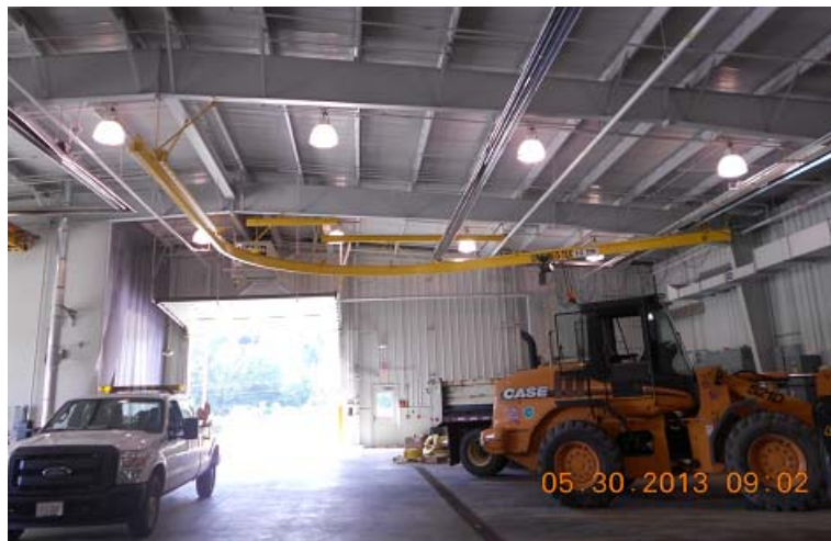
Figure 4.8. 400 W metal halide lamps used in the garage/maintenance area
