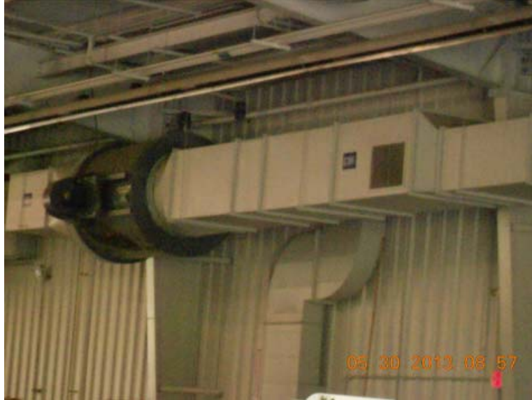
Figure 4.7. Large exhaust fans provide ventilation to maintenance/garage areas
