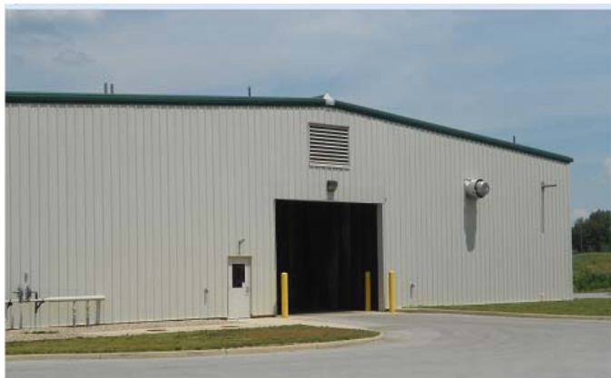
Figure 7.4. South East wall where collector is assumed installed for the Pike County Garage SAH system LCCA
