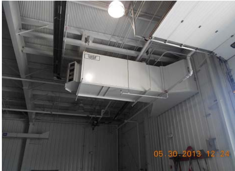
Figure 4.3. Gas fired make up air units provide space heating for the maintenance/garage area
