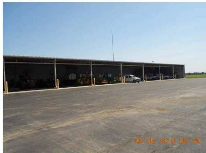
Figure 4.30. The southern wall of Seneca County Garage is shaded by an unconditioned storage area.
