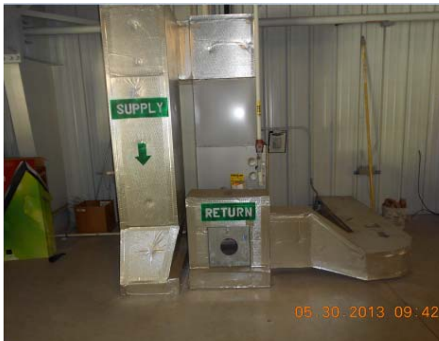
Figure 4.4. Gas fired furnace provide space heating for the office area
