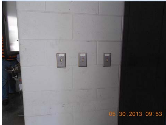
Figure 4.14. Basic on/off switches are used to manually control lighting circuits
