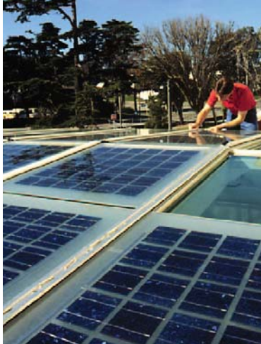
Figure 6.11. Installation of skylight glass laminated with PV cells at the Thoreau Center for Sustainable Development, Presidio National Park, San Francisco, California. (Credit: Lawrence Berkeley Lab)
