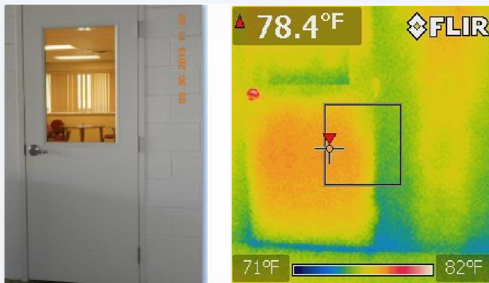
Figure 4.21. Infrared camera shot of a visited facility door displaying temperature differentiation indicating infiltration.
