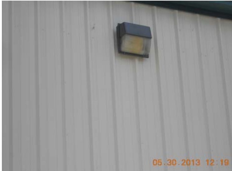
Figure 4.9. Building mounted 175 W metal halide lamps are used for outdoor site lighting
