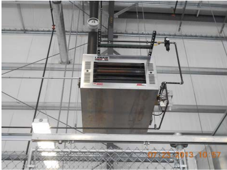
Figure 5.6. Waste oil heater in New Lucas County Garage's maintenance area
