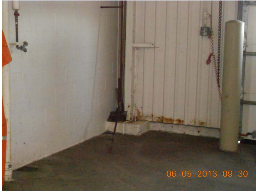
Figure 5.4. Corrosion of structural steel and metal wall in truck washing area
