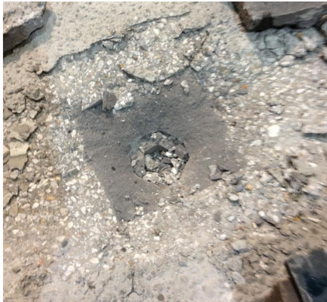
Figure 5.24: Pullout failure mode
