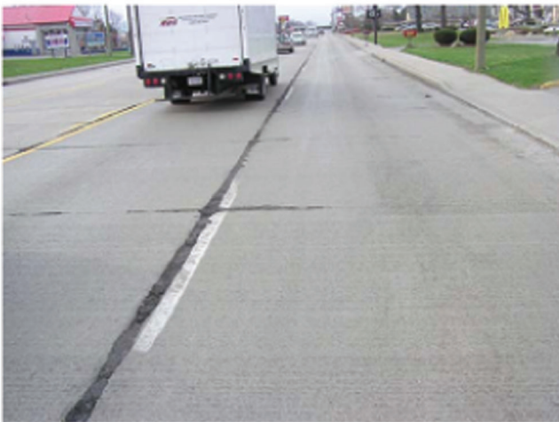
Figure 1.1 Joint deteriorations at section of Indiana State Road SR-933.
