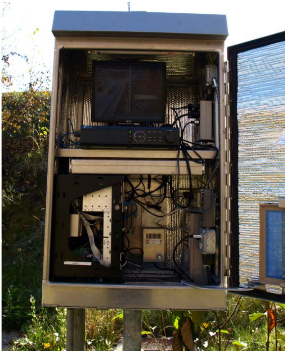
Figure 5 Overheight Detection System Controller Cabinet
