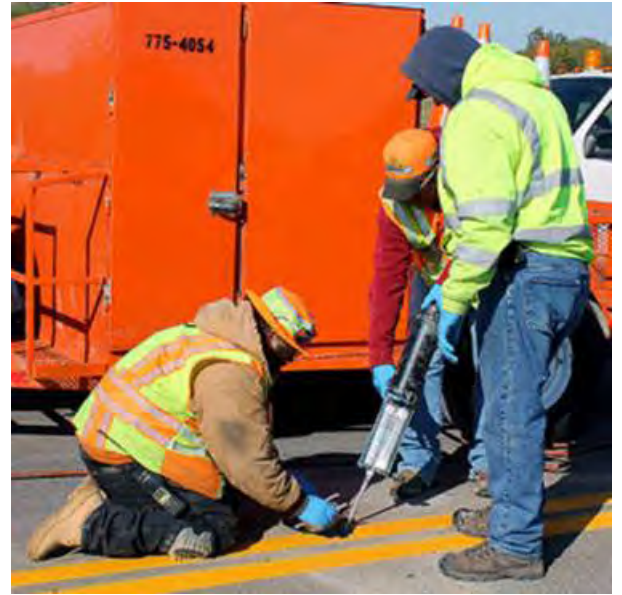
KDOT Workers Install a Solar Powered Light on Old 169 Highway Near the Humboldt-Chanute Road Interchange. KDOT Will Install 110 Lights at That Interchange and 490 at the Plummer Interchange.
