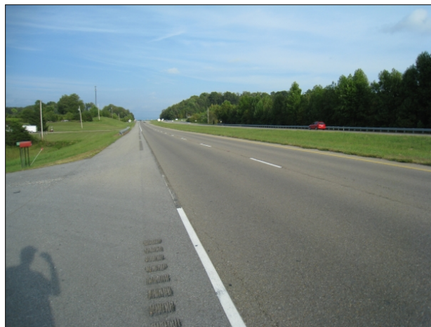
Figure 5. Photo. Tusculum test deck section 5 TN-T b shallow groove-applied presence failures.
