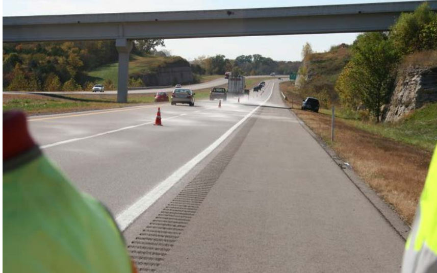
Figure 39. Photo. Glass bead application on a highway on the Tennessee test deck.
