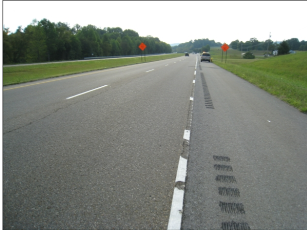
Figure 4. Photo. Tusculum test deck section 5 TN-T a shallow groove-applied presence failures.
