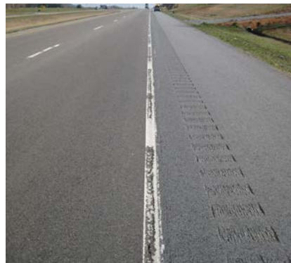
Figure 3. Photo. Tusculum test deck section 1 TN-T presence failure.
