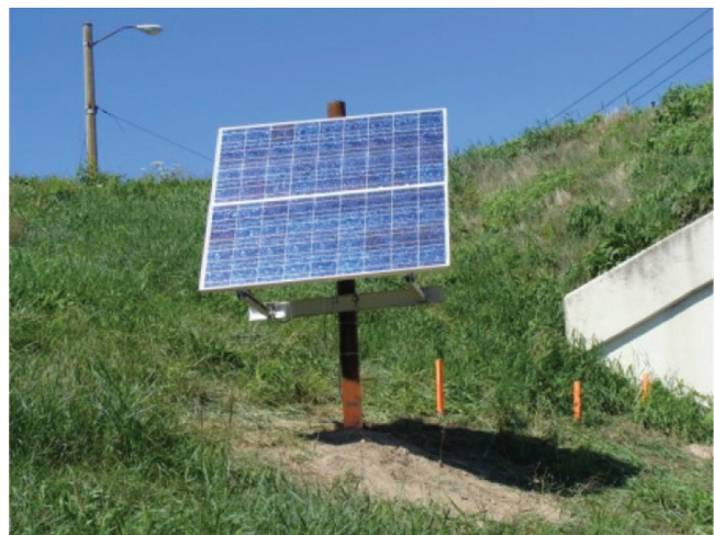
Figure 4.7 Solar panel assembly used to recharge the battery system.
