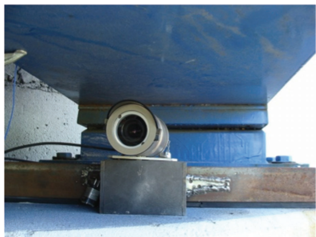
Figure 4.4 Campbell Scientific CC5MPX digital network camera installed beneath the bridge girder.
