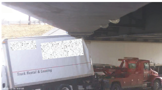
Figure 5.1 Still image taken from HD video footage of a truck impacting the northern girder of the Virginia Avenue Bridge over I-65 SB (note date and time stamp in lower left of image).
