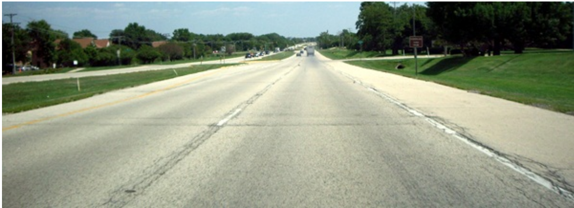
Figure 1. Pavement surface condition before construction.
