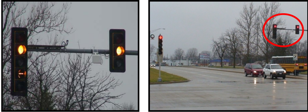
(a) Wavetronix Matrix on westbound mast arm overlooking the stop bar zones of eastbound lanes
