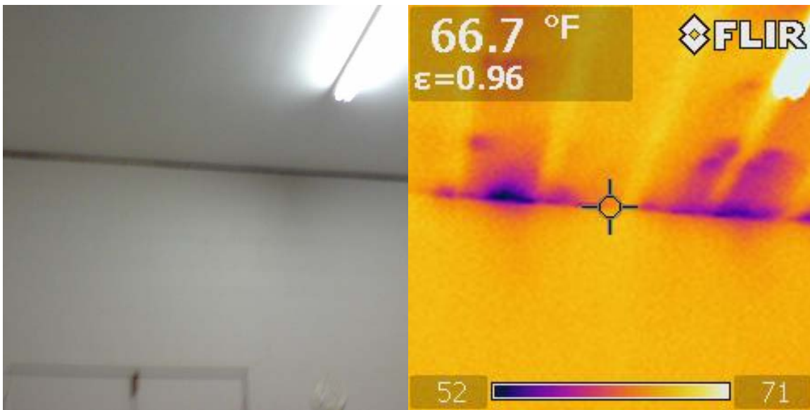
FIGURE 4.27 Infiltration Detection—Wall and Ceiling Seam
