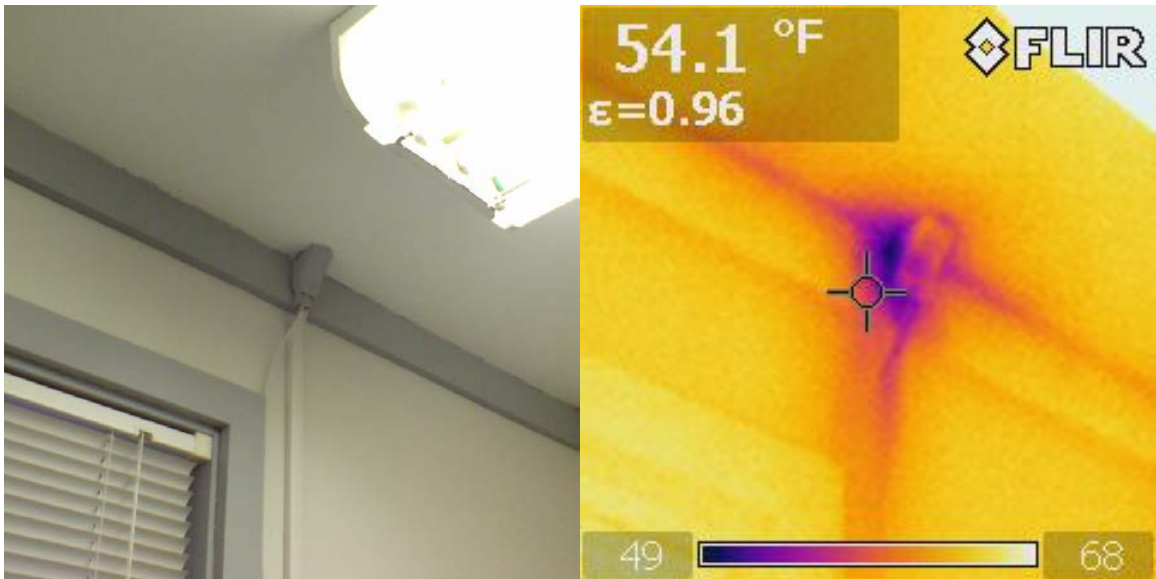
FIGURE 4.24 Infiltration Detection—Ceiling Penetration
