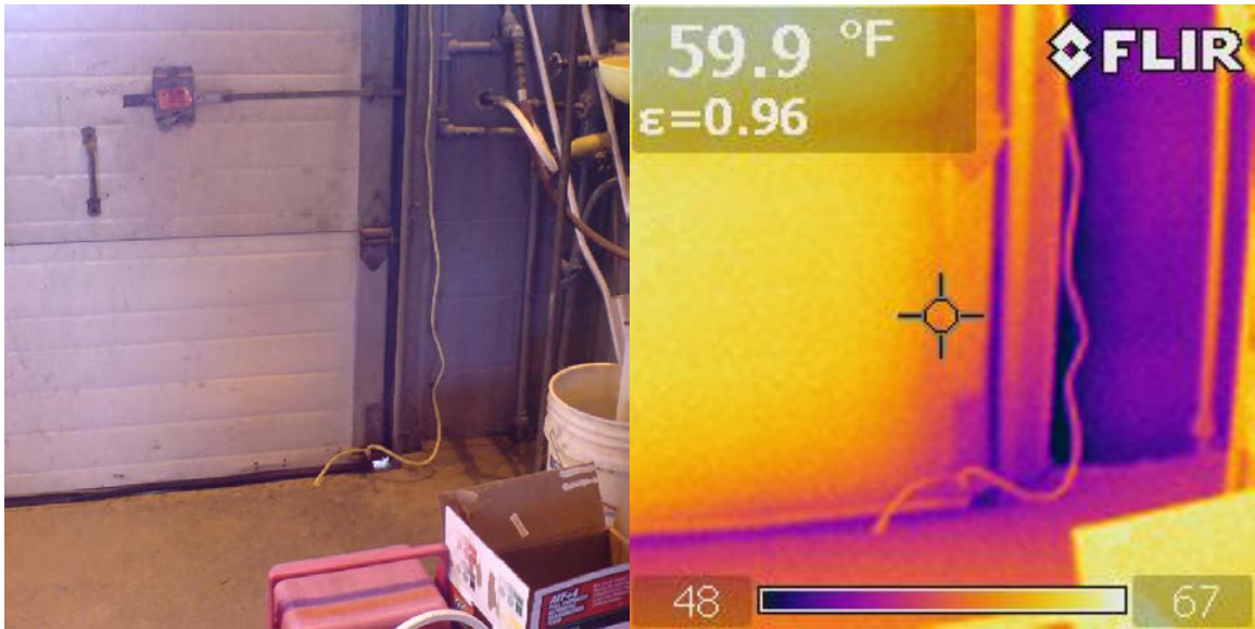
FIGURE 4.35 Infiltration Detection—Bay Door
