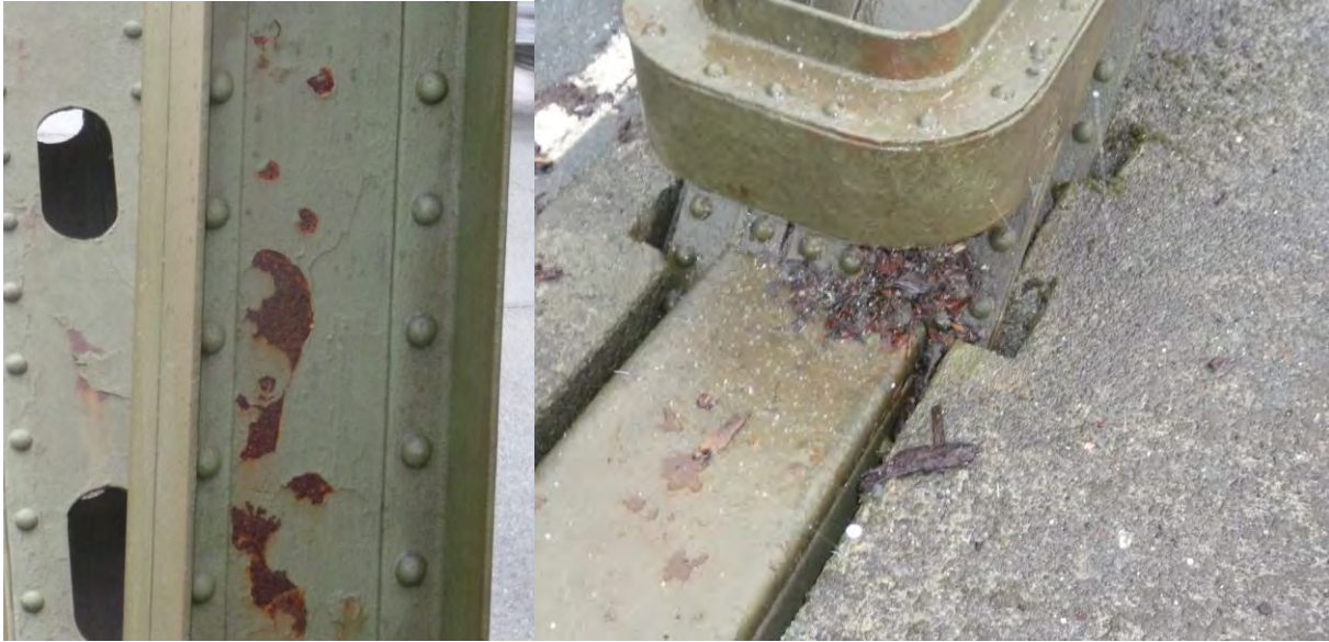
Figure 5. Sol Duc #5 Bridge with rough paint surface and problem area where girder meets the deck
