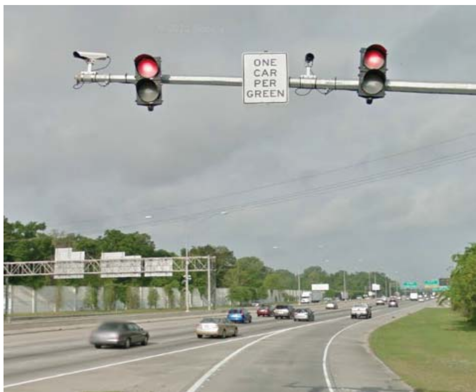
Ramp meter on I-12 at Essen Lane
