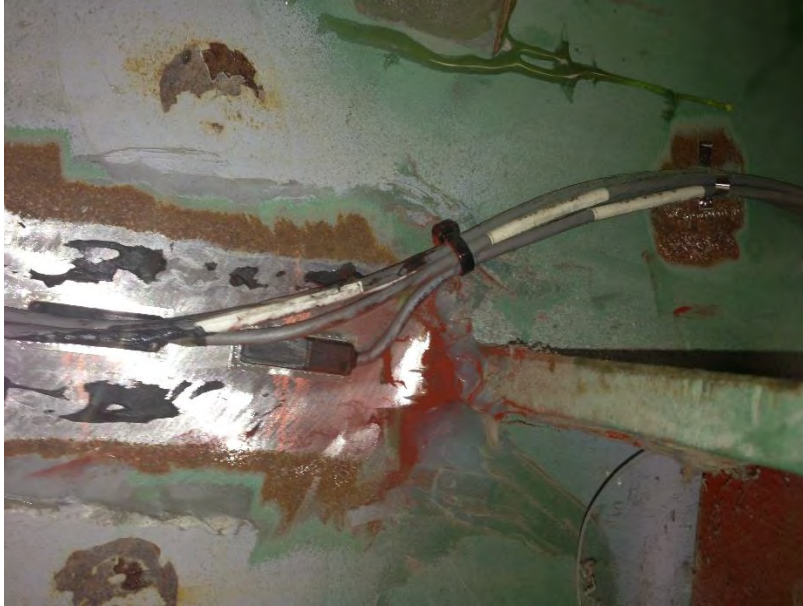
Figure 4.10. Photograph of a potential fatigue crack in web cut-back region
