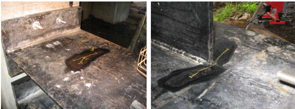
Figure 2.6. Sacrificial Specimen 1 cracking (Phares et al. 2011)
