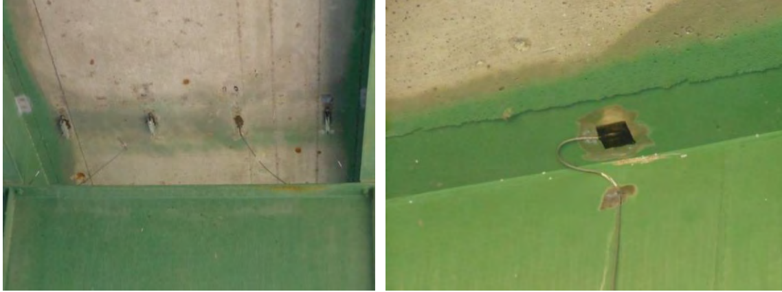
Figure 3.6. Deck bottom sensors (left) and sensor installation sample on top flange of girder (right)
