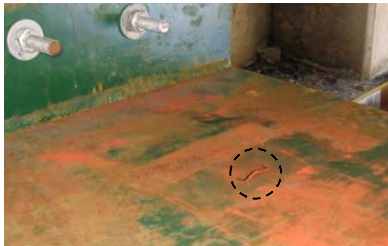
Figure 2.8. Sacrificial Specimen 2 top web plate cracking (Phares et al. 2011)
