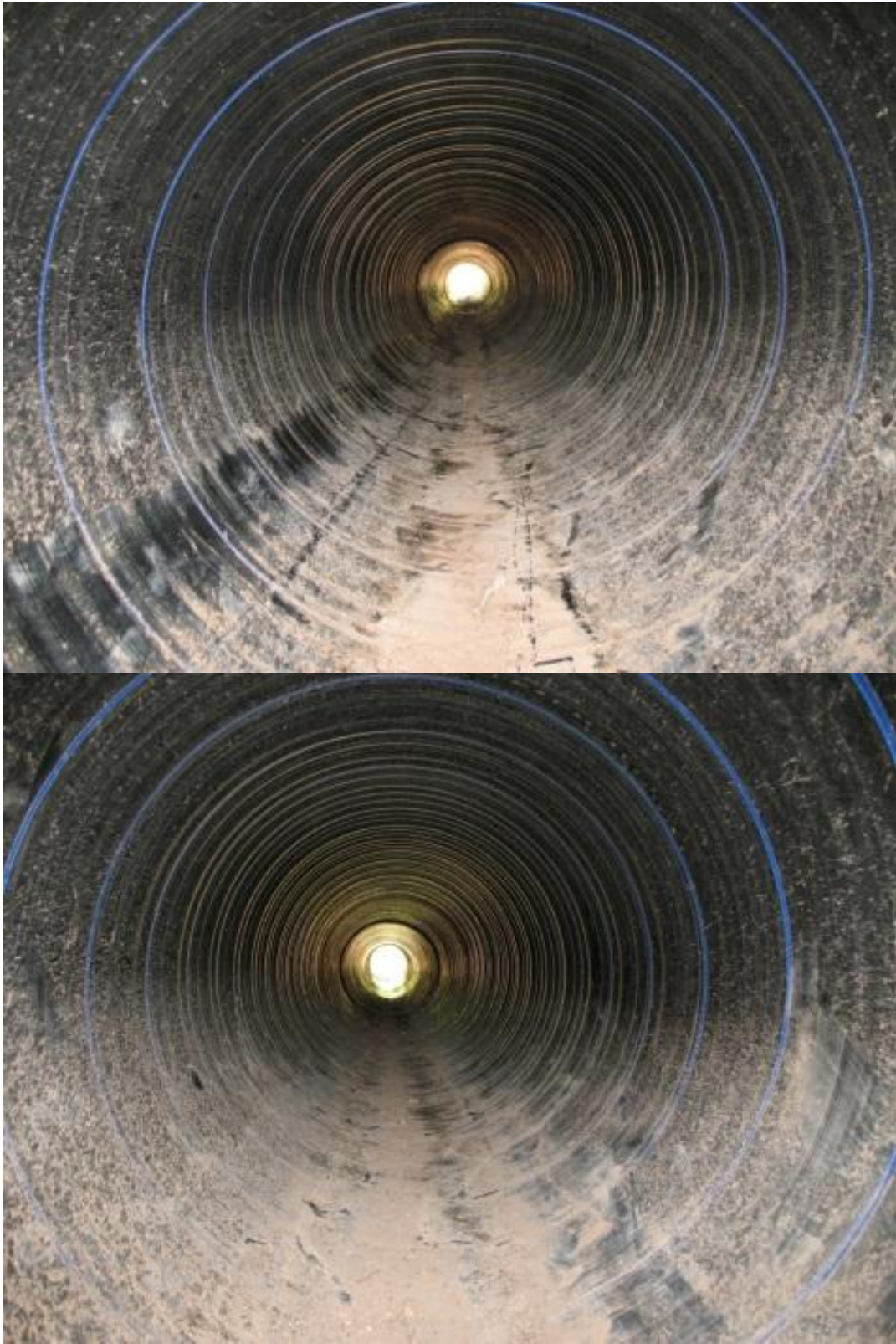
Figure 8. DuroMaxx pipe photos after 1 year; north pipe (top) and south pipe (bottom).
