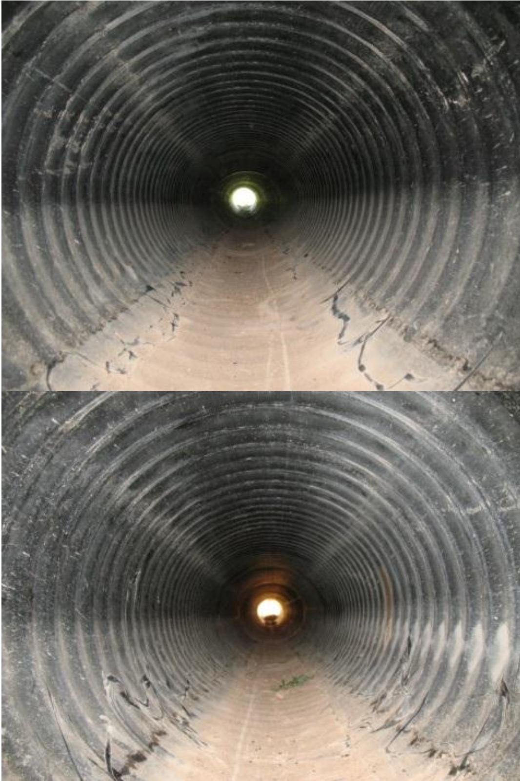
Figure 13. ADS pipe photos after 3 years; north pipe (top) and south pipe (bottom).
