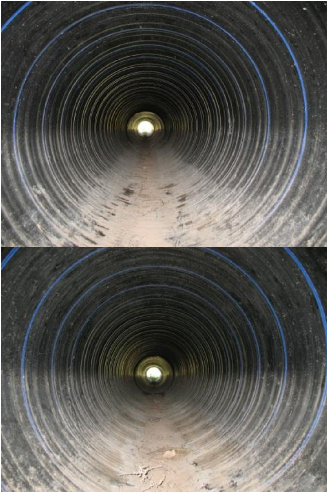
Figure 12. DuroMaxx pipe photos after 3 years; north pipe (top) and south pipe (bottom).
