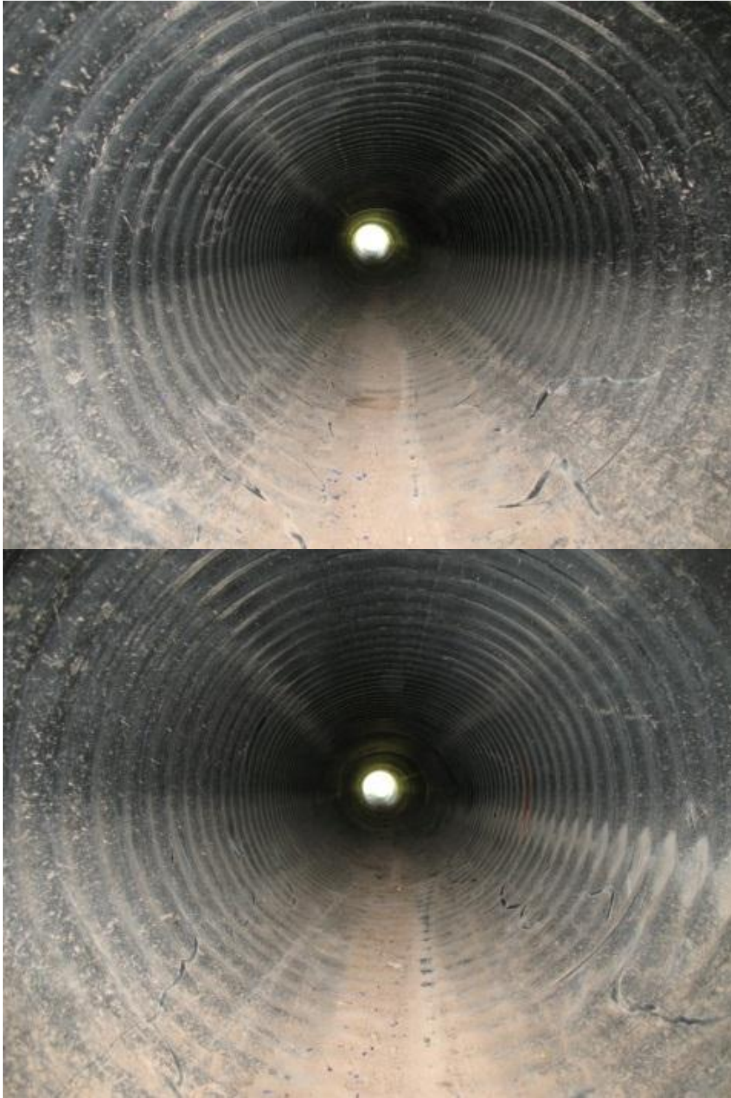
Figure 11. ADS pipe photos after 2 years; north pipe (top) and south pipe (bottom).
