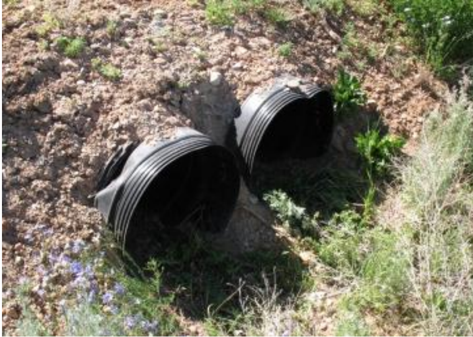
Figure 16. Damage to the west entrance to the DuroMaxx pipe.
