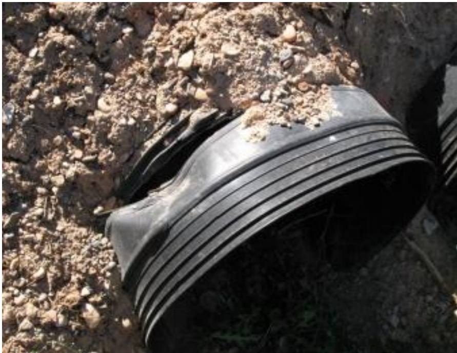
Figure 17. Close up view of damage to the west entrance to the north DuroMaxx pipe.
