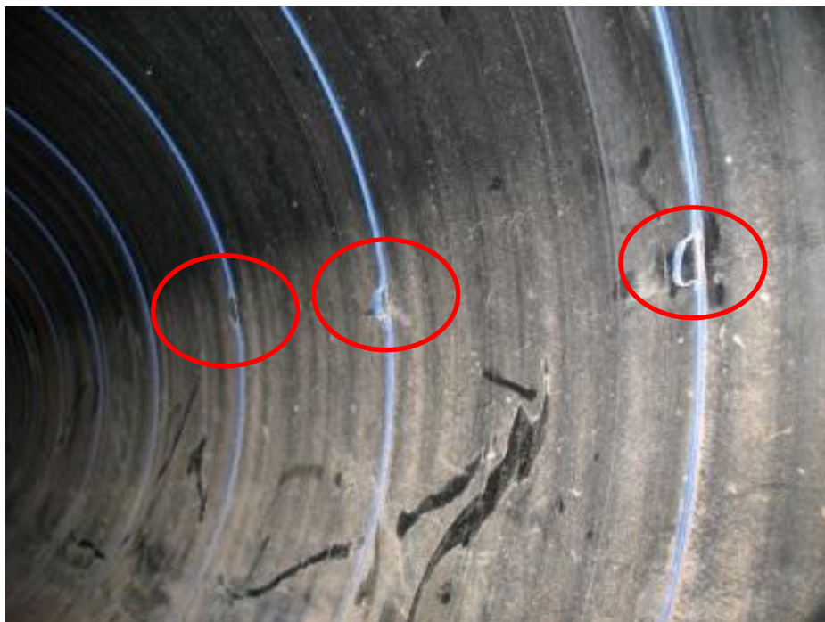
Figure 15. Minor damage to plastic seal at spiral weld locations.
