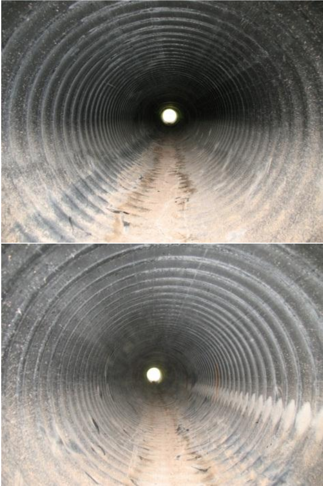
Figure 9. ADS pipe photos after 1 year; north pipe (top) and south pipe (bottom).
