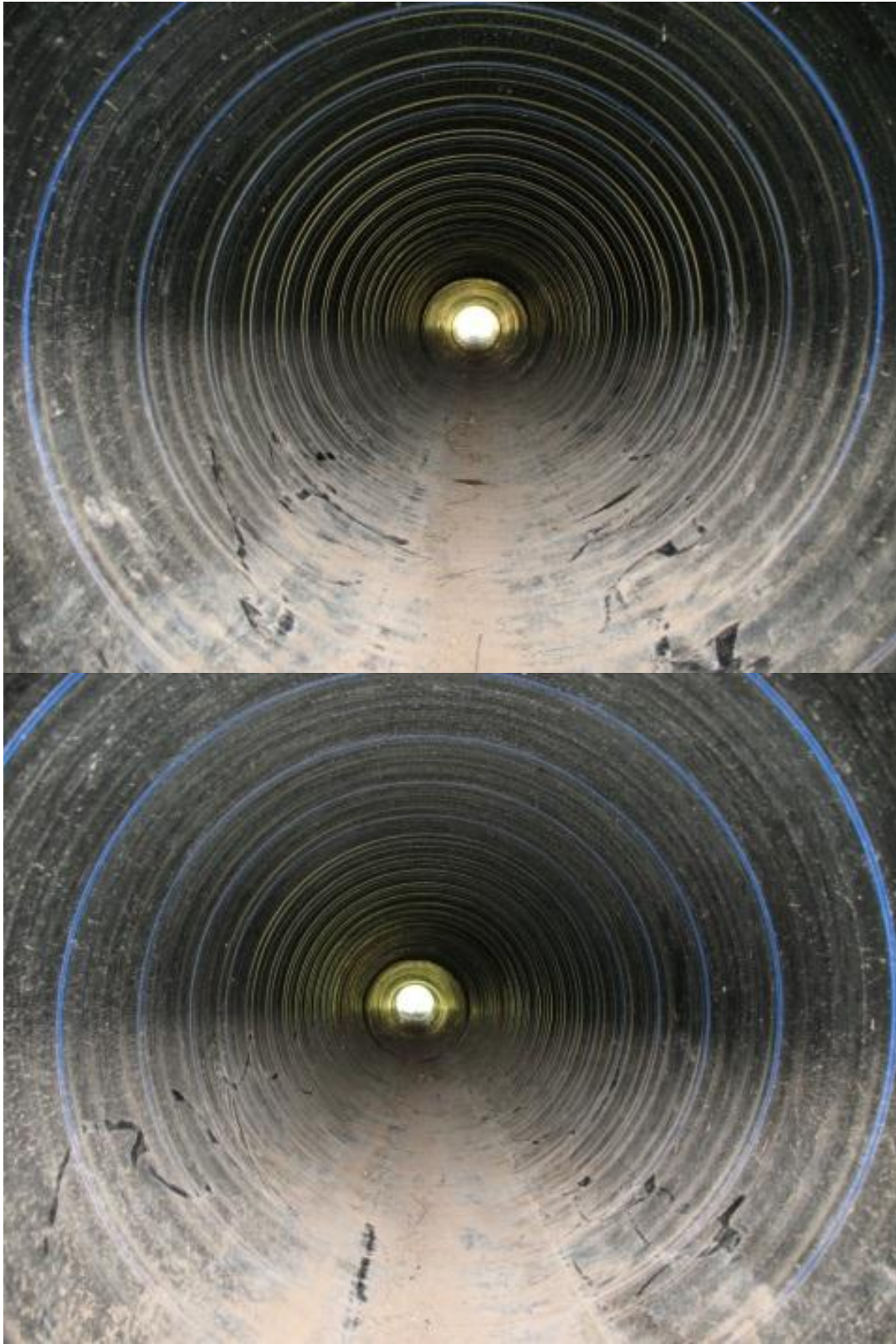
Figure 10. DuroMaxx pipe photos after 2 years; north pipe (top) and south pipe (bottom).
