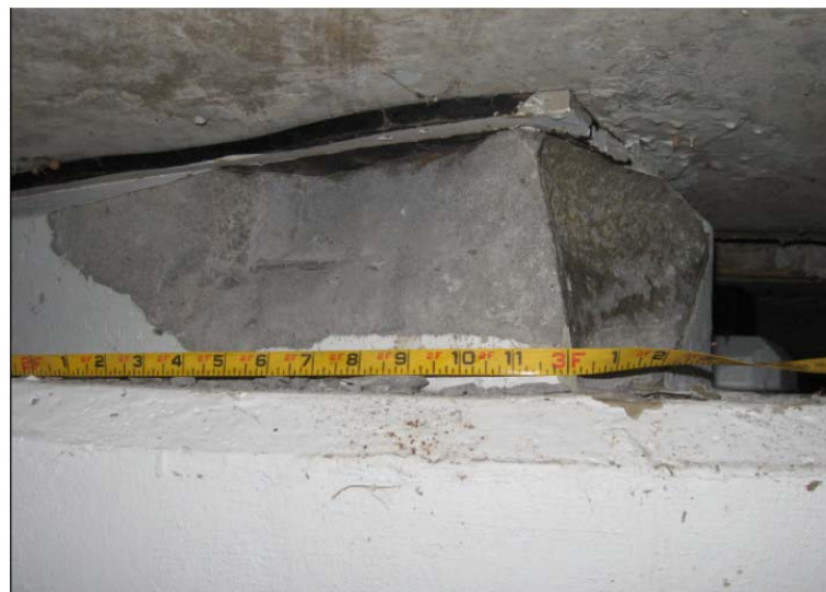
Figure 3-6: Spalled Portion of the Pedestal 12 at the Pier 2 in the Bridge 1026170.
