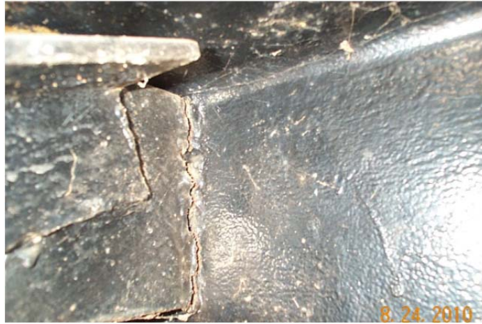
Figure 4-6: Photograph of Cracked Diaphragm Bracing Connection.
