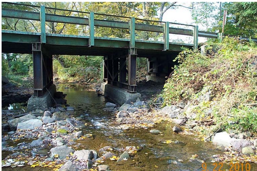
Figure 4-9: Elevation View of Bridge 3350660 Showing Footings Exposed to Scour.
