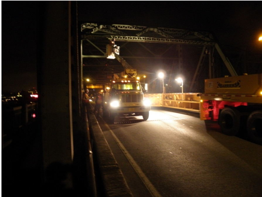
Figure 3.10: Workers Repairing Electrical Circuits on I-5 Interstate Bridge with MBT-1® (Case Study #3)
