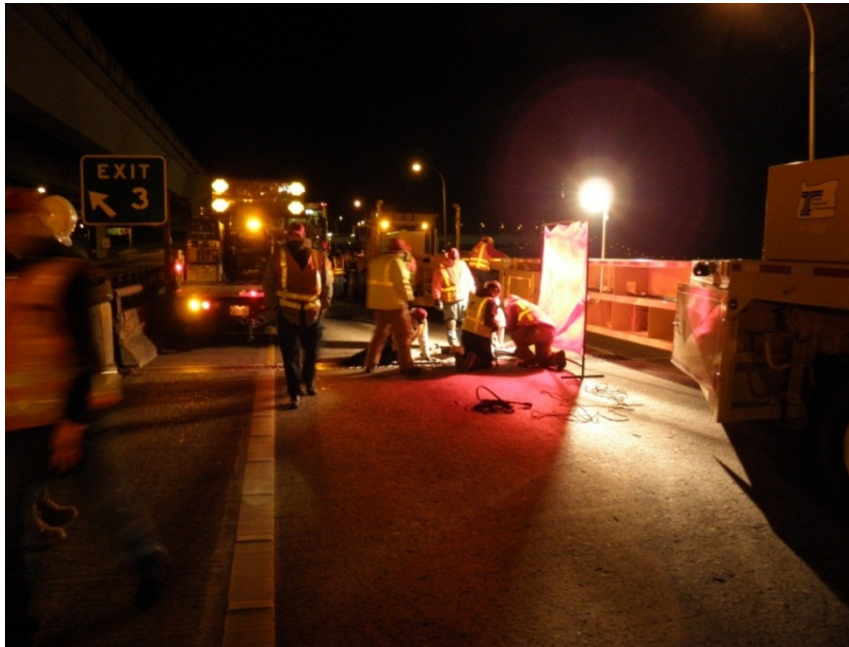
Figure 3.3: ODOT Bridge Crew Working on Repair of Fremont Bridge Joint with the MBT-1® (Case Study #1)
