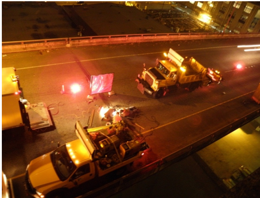
Figure 3.4: ODOT Bridge Crew Working on Repair of Fremont Bridge Joint without the MBT-1® (Case Study #1)
