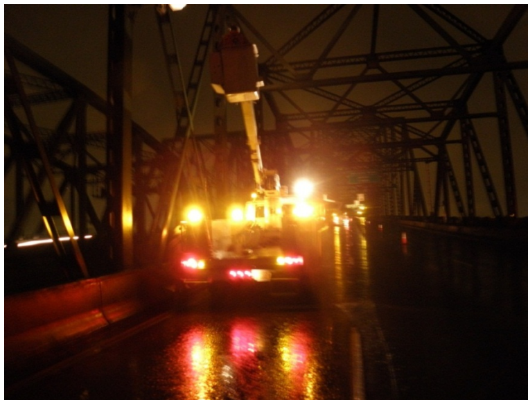
Figure 3.7: Crew Repairing Lights on I-5 Interstate Bridge without the MBT-1® (Case Study #3)
