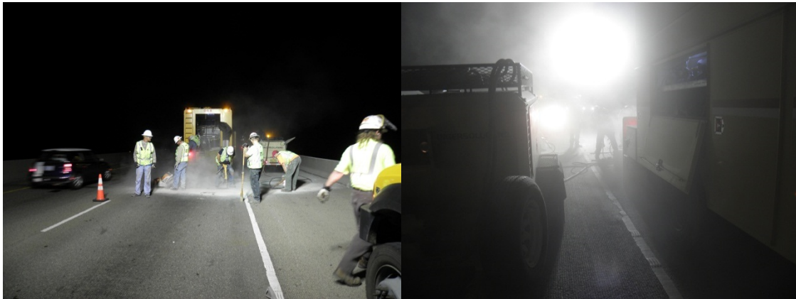
Figure 3.18: Jackhammering and Concrete Cutting (left); Dust from Concrete Cutter 'Fogging' Work Area (right) (Case Study #6)
