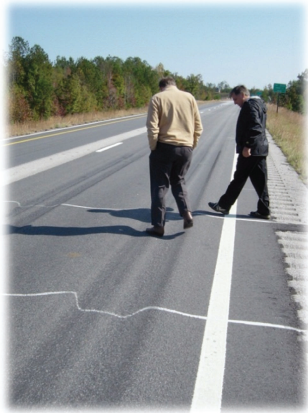
Figure 4.2 Severe rutting before reconstruction.
