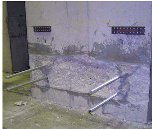
(b) Failed abutment concrete
