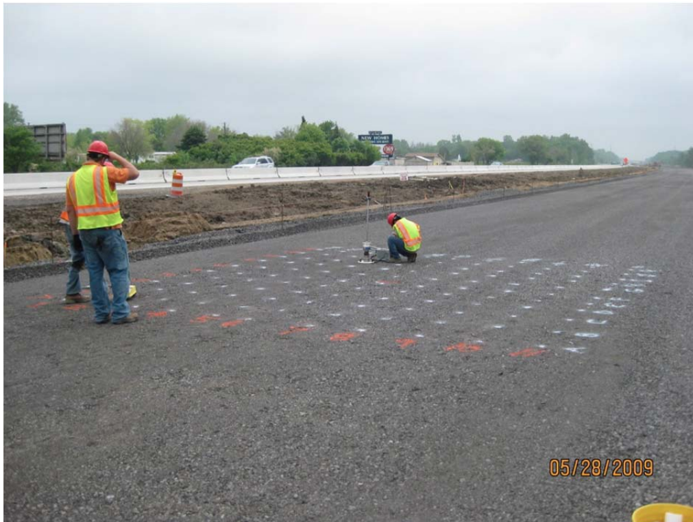
Figure 39. DCP test being carried out on an OGDC layer on TB1b. Source: White et al. (2011)
