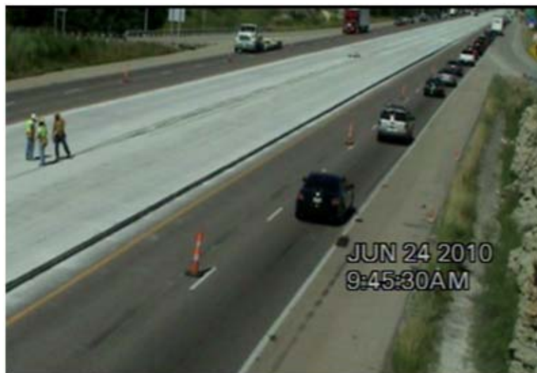
Figure 3.1 Work Zone View from a Data Collection Camera, Interchange at Mile Marker 253, I-44 WB
