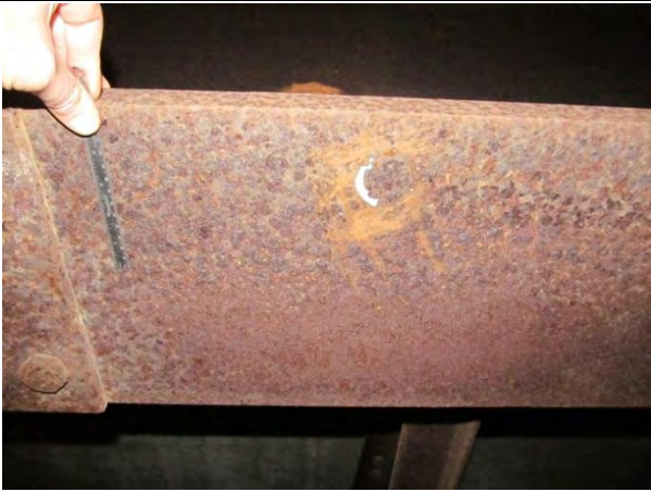
Figure 3. Heavy flaking (Index = 2) on bottom of west fascia bottom flange over shoulder.
