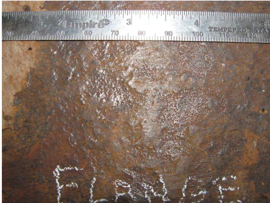
Figure 33. Close-up photo of steel on top surface of girder bottom flange after wire wheel grinding at Field Selection 3; delaminated patina removed down to bare steel with oxide layer remaining in pitted areas.
