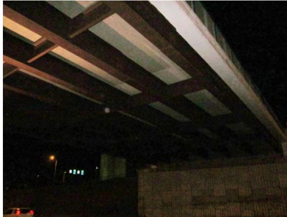
Figure 1. South span over eastbound I-235. Some staining noted on fascia girder and 1st interior girder over the center lane, but not readily visible in this photo.
