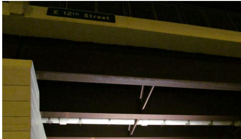
Figure 1. White, salty staining on west fascia girder (toward oncoming traffic) bottom flange south of pier.
