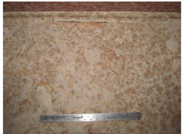
Figure 6. Delaminated, heavy pultice corrosion on interior bottom flange.
