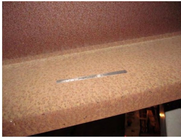
Figure 3. Light poulitice corrosion without flaking or deterioration on fascia girder flange.
