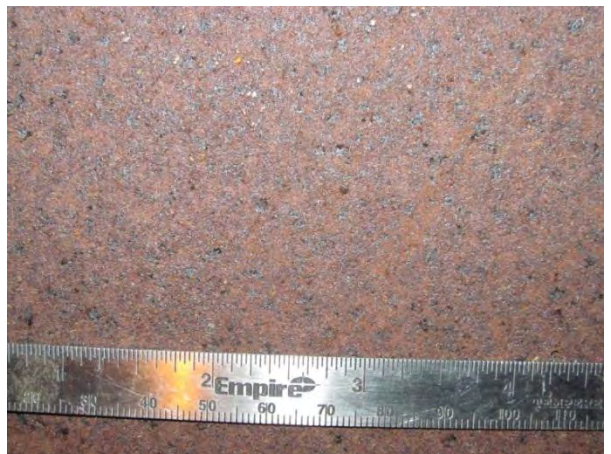
Figure 6. Detail of patina condition on diaphragm web adjacent to core. Index=3.5.
