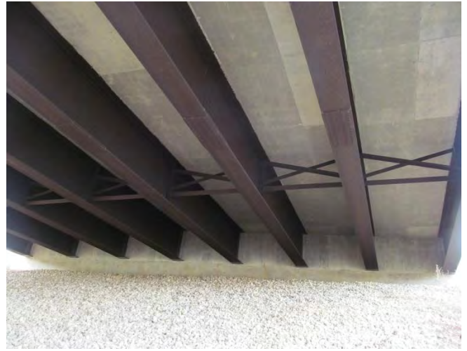
Figure 2. Typical conditions underneath interior of both bridges. Index = 3.5 to 3 on bottom flanges. Sound deck prevents water infiltration from above.
