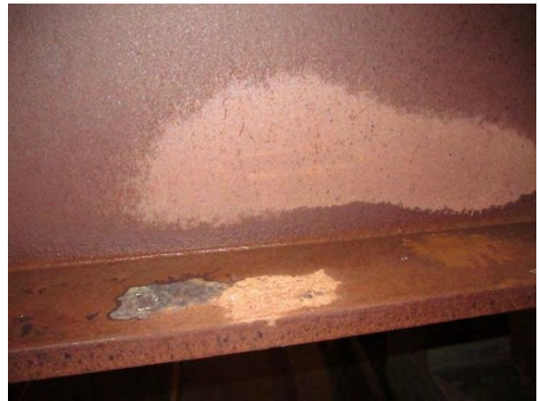
Figure 4. Test area after washing and partial drying: wire wheel area on left, wire brush area on far right.
