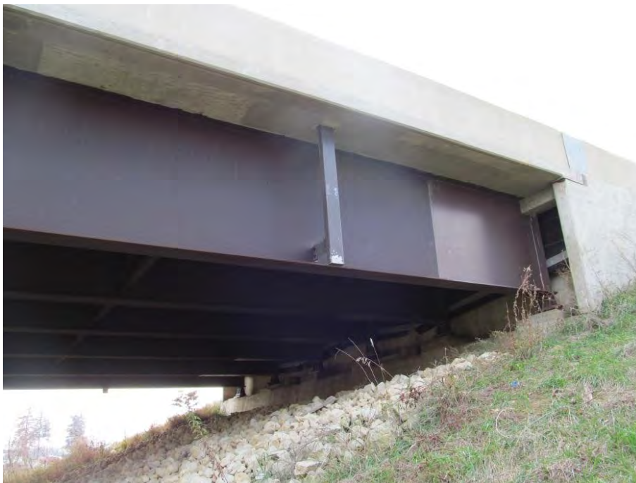
Figure 15. Typical detailing for weathering steel bridges in Iowa, note the painted ends of the girder.
