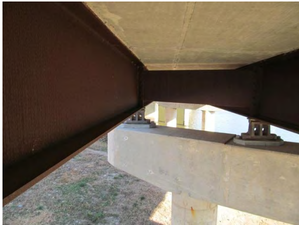
Figure 3. Interior side of entrance ramp north fascia girder demonstrating good patina performance.
