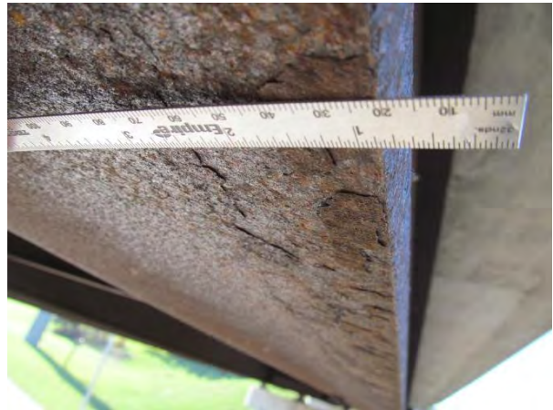
Figure 2. Bottom of bottom flange delaminations, north fascia girder of entrance ramp.
