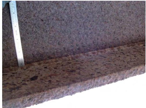
Figure 2. Interior surfaces over traffic showing signs of long-term deterioration.
