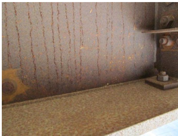
Figure 3. Interior girder over traffic showing poultrice with minimal flaking and reddish web discoloration, possibly due to mill scale.
