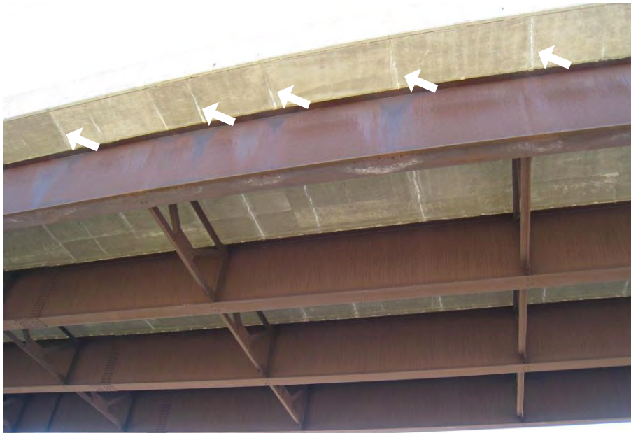
Figure 35. Cracking with efflorescence noted in the concrete deck (arrows) at Structure 9799.5L075, Field Selection 10. Note areas of non-uniform, black weathering steel patina and salt staining on the bottom flange below each crack in the deck.
