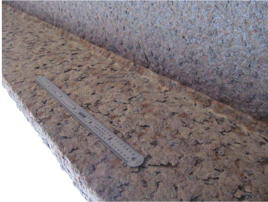
Figure 20. Category 1 patina on top of an interior girder bottom flange; note the large, loose, thick flakes that cover virtually the entire surface. Section loss is not yet apparent in this case.
