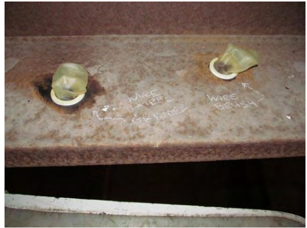
Figure 2. Chloride tests with some leaking on chalky poutlice of bottom flange before washing.
