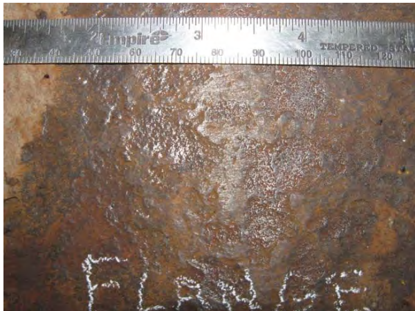
Figure 3. Top of bottom flange ground with wire wheel. Chlorides in ground area before washing = 20 ppm; after washing, 14 ppm extracted by test.
