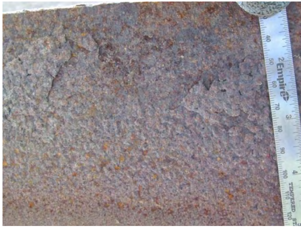
Figure 3. Close up of delaminations and discoloration of bottom of fascia girder bottom flange.
