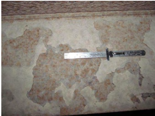
Figure 1. Heavy poultrice on interior flange with multiple thin layers of delamination forming.
