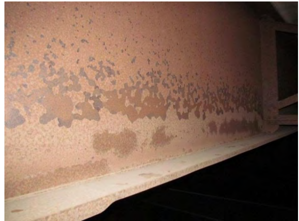
Figure 2. Typical widespread delamination on web above traffic. Lower delaminations appear older, beginning to deteriorate again.
