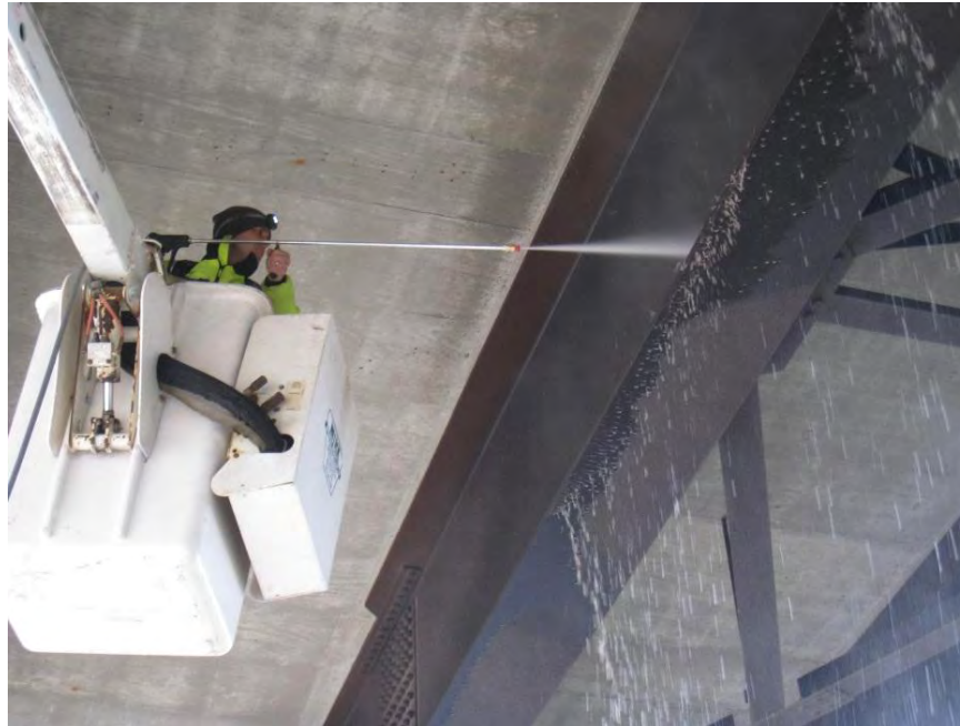
Figure 34. Pressure washing (0° nozzle) on an interior girder of Structure 0819.6R930, Field Selection 1, eastbound Iowa Route 930 over U.S. Highway 30.
