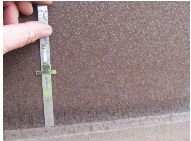
Figure 2. Fascia girder exterior web patina over traffic (Index = 4). Note darker band above weld.
