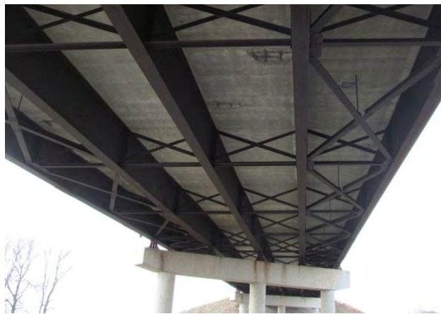
Figure 1. North roadway span showing bracing arrangement and spall locations in the deck.
