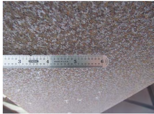
Figure 4. Interior bottom flange condition near north abutment; index here is 3.5. Contrast with Figure 3 from identical location at south end.
