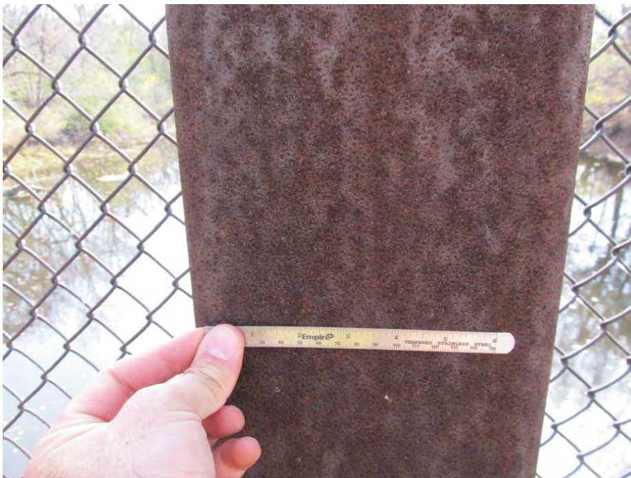
Figure 7. Close-up photo of patina performance on the Des Plaines River pedestrian bridge; patina is dense and adherent, with small constituent rust particles.
