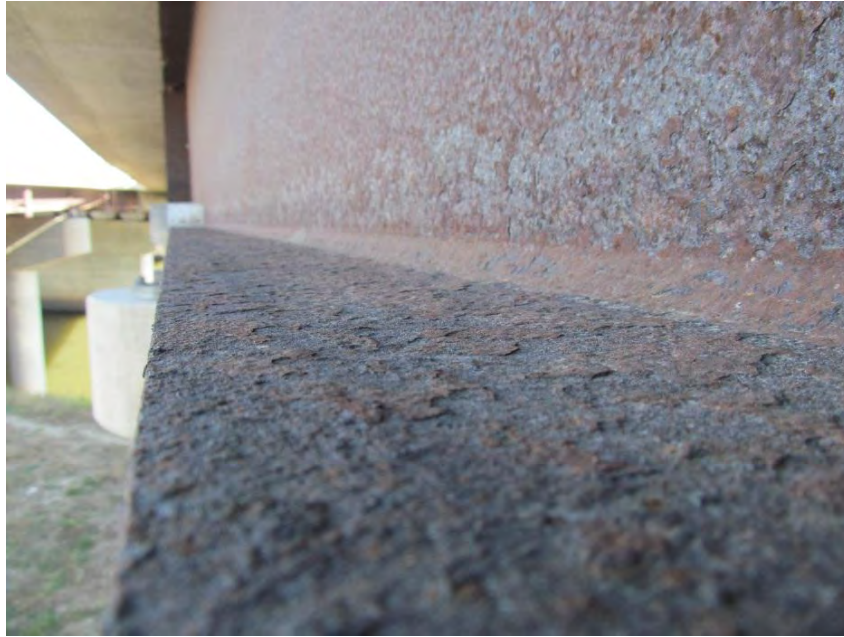
Figure 28. Fascia girder of I-235 eastbound on-ramp at 2nd Avenue. Note transition from Category 3 patina at mid-height of the web to Category 2 at the top of the bottom flange in areas subjected to direct salt spray from the I-235 mainline.
