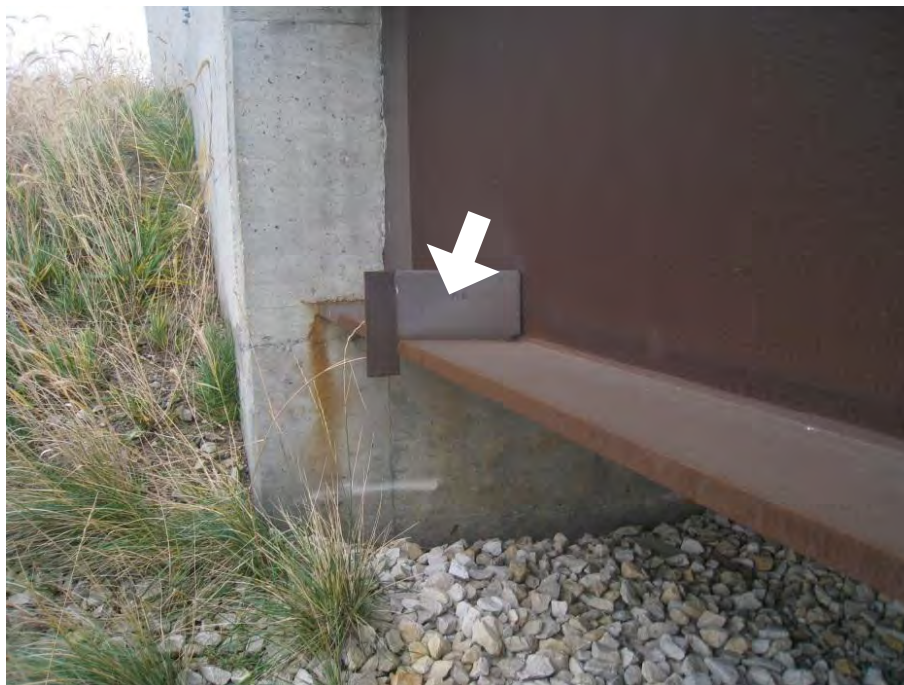
Figure 13. Typical detailing for weathering steel bridges in Iowa, note the water diversion plate (arrow), the painted ends of the girder, and the use of integral abutments.
