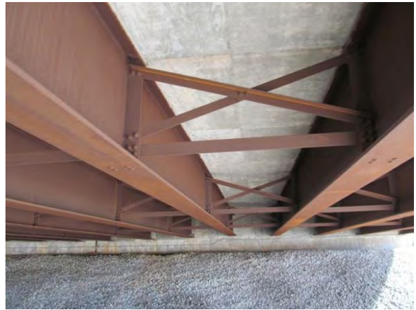
Figure 2. Some discoloration on bottoms of flanges, but only minor flaking. Conditions near abutment similar to those over traffic.
