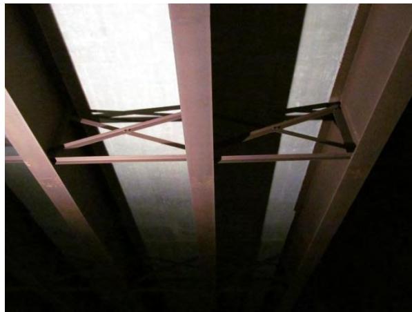
Figure 2. More distinct spots of local discoloration visible near middle of south span.
