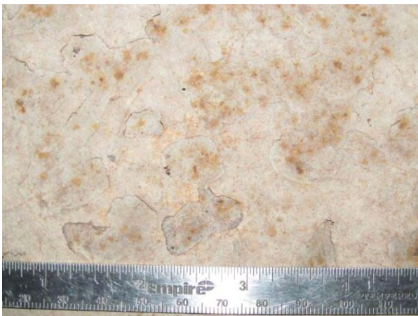
Figure 5. Delaminating patina with heavy poultrice corrosion on interior girder bottom flange.
