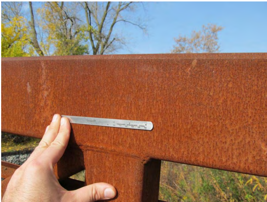
Figure 5. Developing patina on pedestrian bridge in a suburban Illinois park. Note the adherent, small size of the patina rust particles, and the reddish coloration.
