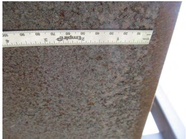
Figure 4. Larger flakes on bottom of fascia bottom flange near downspout by south abutment.
