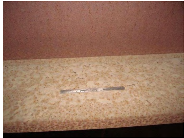
Figure 4. Heavy poulitice corrosion with delaminated flaking on interior bottom flange.
