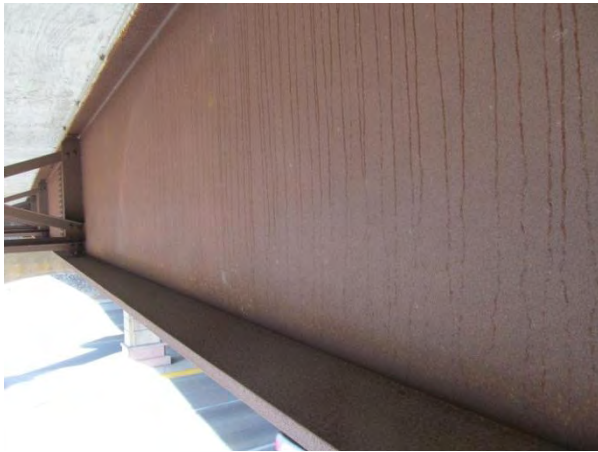
Figure 1. Typical interior girder conditions; good patina performance on web and flange, despite flange poutlice.
