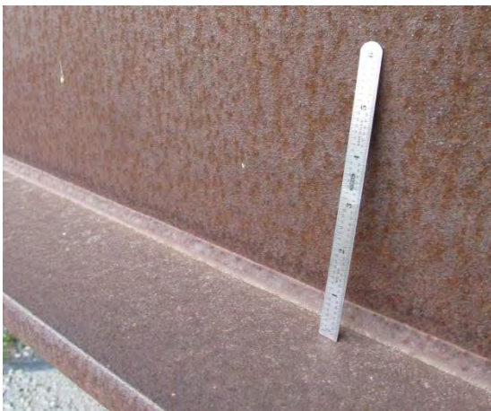
Figure 5. Excellent patina performance on exterior fascia faces after 40 years, typical of rural bridges.
