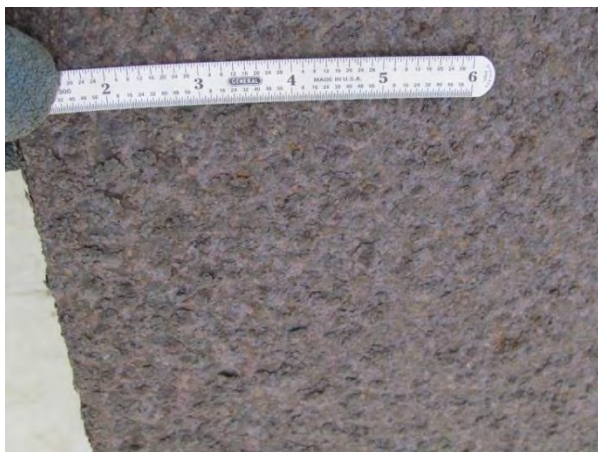
Figure 5. Heavy flaking of bottom of flange in traffic span, typically Index = 2 or worse.
