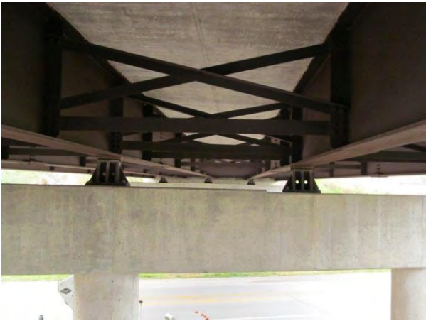
Figure 1. View of south pier looking north; note lack of drainage deflector plates on bottom flanges, typ.
