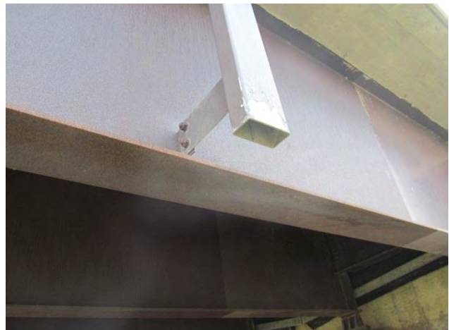
Figure 6. View of downspout; bottom flange corrosion extends away from spout, primarily in direction of girder slope.
