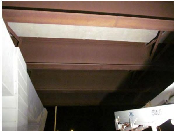
Figure 1. Bottom flanges exhibiting some mild reddish discoloration and possible flaking near pier over eastbound left shoulder.
