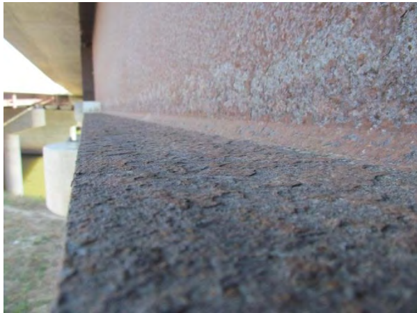
Figure 1. Delamination of top of exterior bottom flange and web of north fascia girder on I-235 eastbound entrance ramp.
