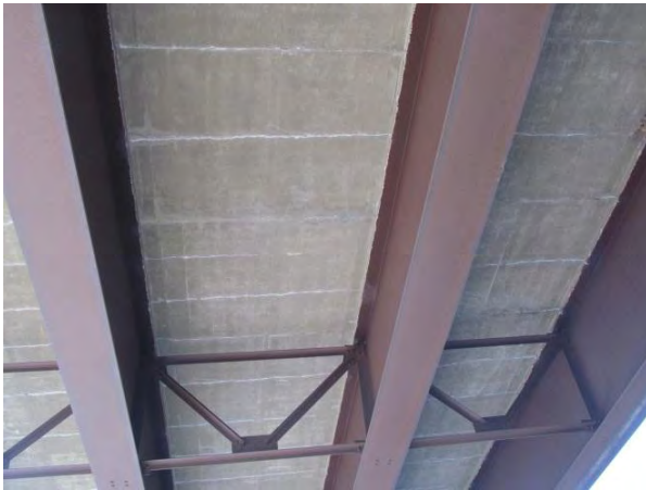
Figure 3. Other girders of southbound bridge show little change in patina condition beneath cracks.
