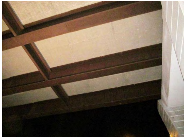
Figure 2. Girders and diaphragms near south pier; appear in good condition from below.
