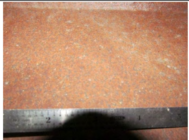
Figure 6. Washed area of top of flange patina after fully dried; adherent, well-behaved beneath chalking.
