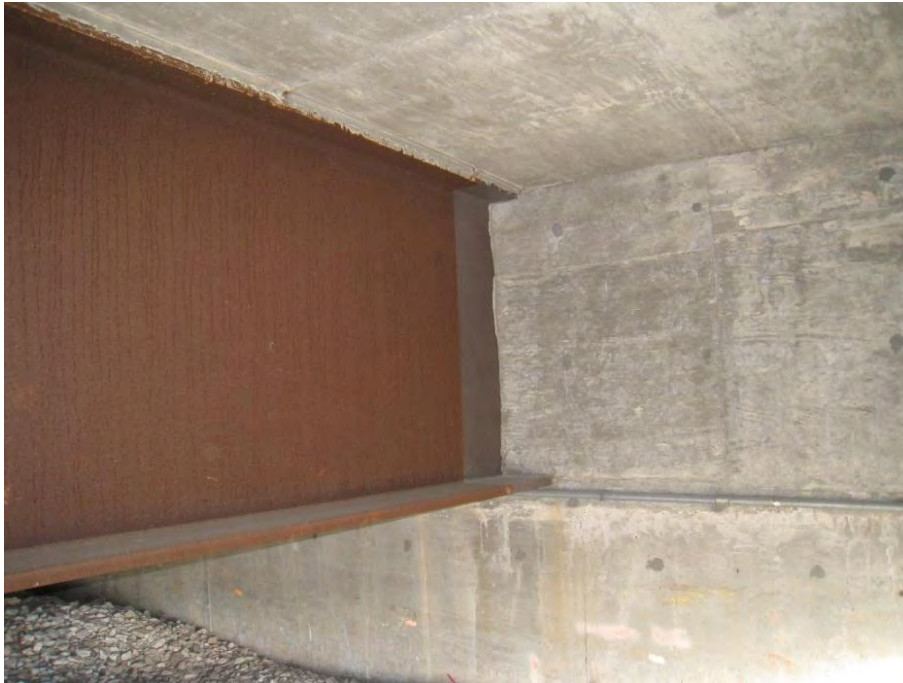
Figure 14. Typical detailing for weathering steel bridges in Iowa, note the use of integral abutments and the painted ends of the girder.
