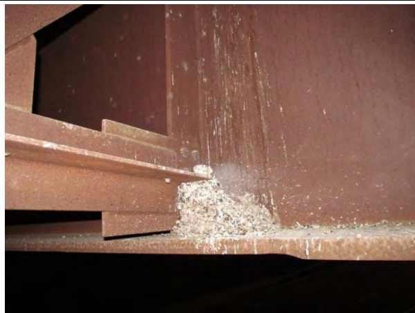
Figure 5. Bird droppings contributing to poulitice on interior bottom flange.
