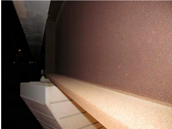
Figure 1. Index = 3.5 to 3 patina on exterior fascia surfaces.
