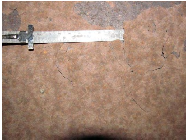
Figure 3. Close-up of web delamination progressing with scale inserted behind loose flake
