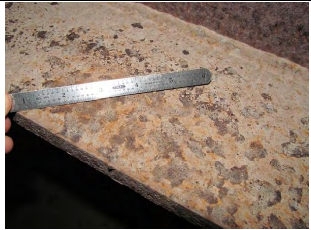
Figure 4. Delamination of interior girder bottom flange with heavy poultice subjected to light scraping.
