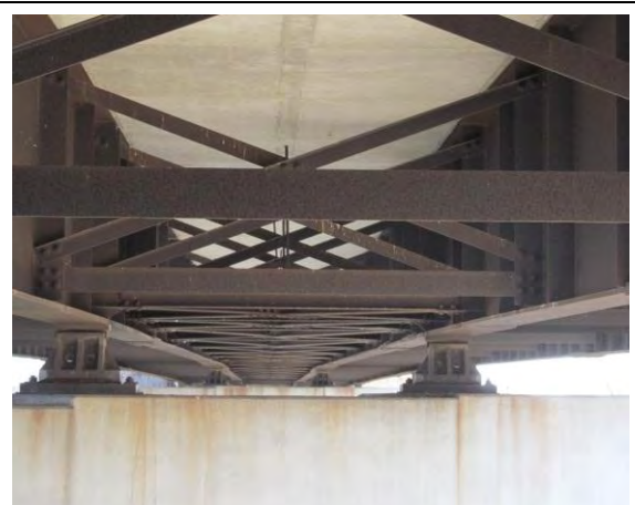
Figure 6. Center bay viewed over top of south pier; note lack of deflector plates and concrete staining.
