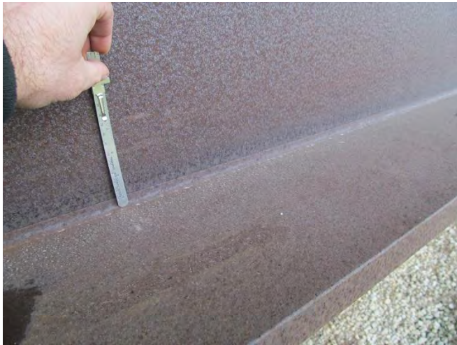
Figure 3. Index 4 and 3 patina on web and top of bottom flange, respectively, near fascia girder tape and chloride tests on 608020.
