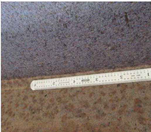
Figure 3. Interior surfaces near east abutment with less deterioration than areas over traffic.
