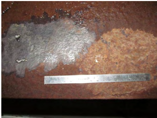
Figure 3. Close-up of wire wheel ground area and adjacent as-is poutlice after washing and drying.
