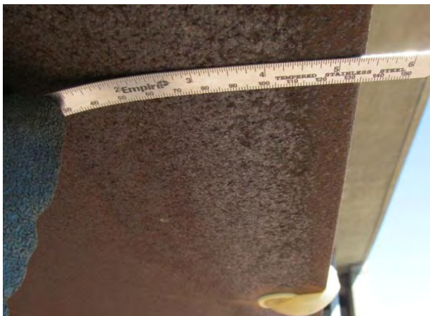
Figure 5. Condition of bottom of flange of east fascia near north abutment considerably better than west fascia (Index = 3).
