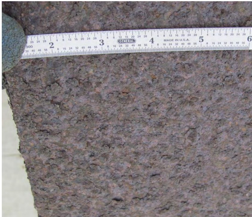
Figure 19. Close-up photo of typical Category 2 patina on the underside of an interior girder bottom flange. Medium size flakes are easily peeled away with a fingernail.
