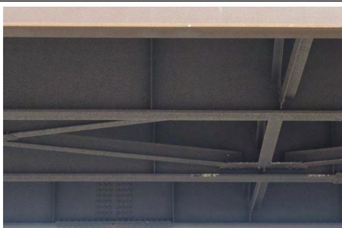
Figure 5. Heavy flaking visible from the ground on interior flanges and webs over traffic lanes; Index = 2.
