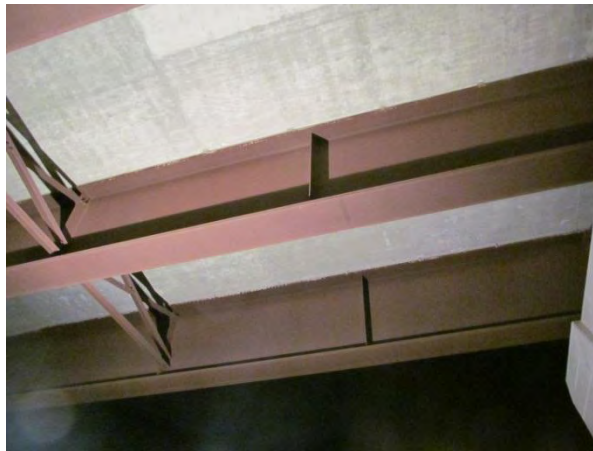
Figure 2. Girders and cross-frames near center pier; no significant deterioration visible from below.
