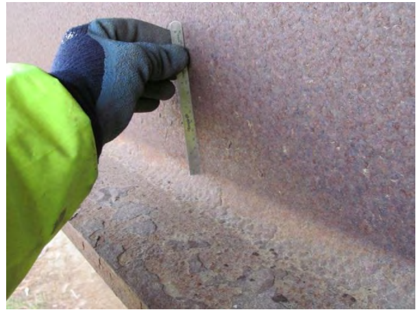
Figure 2. Heavy delamination of fascia bottom flange top (without poulitice); also flaky on web.
