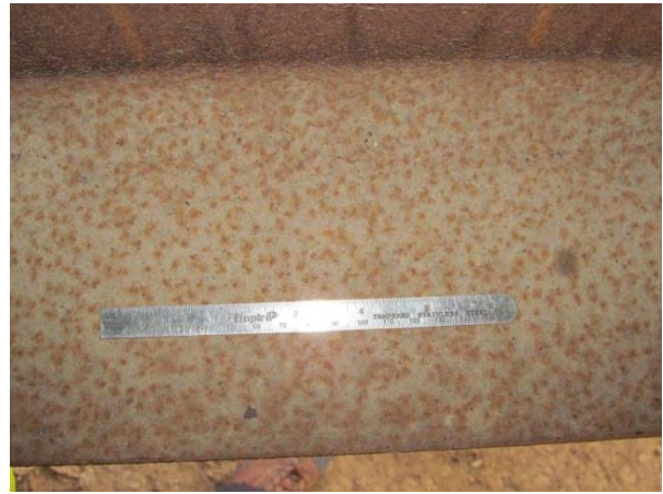
Figure 4. Interior top of bottom fascia flange with light poulitice corrosion, but minimal flakiness.
