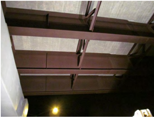
Figure 1. East half of bridge girders near pier; generally good patina condition viewed from below.
