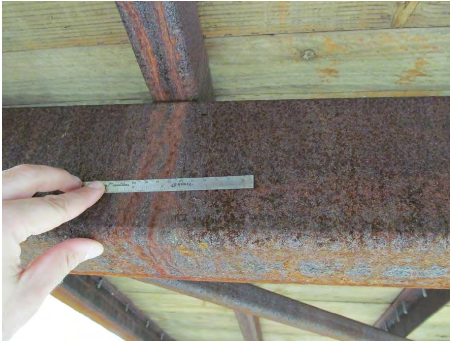
Figure 4. Apparent nonprotective patina on the floor beams and bottom chords of this 10 month old wood-decked pedestrian bridge.
