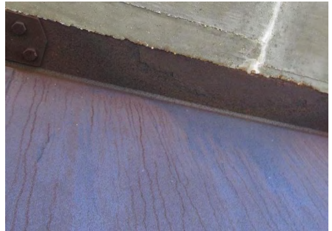
Figure 4. Heavy deterioration/delamination of west fascia girder top flange at crack, possibly Index = 1.
