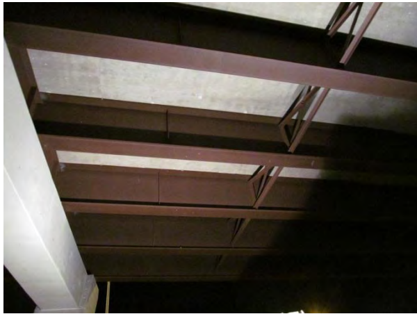
Figure 1. Overall condition of girders and bracing viewed from below, here near pier.
