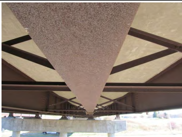
Figure 5. Bottom of flange near west abutment shows less flaking than east side; Index = 3.
