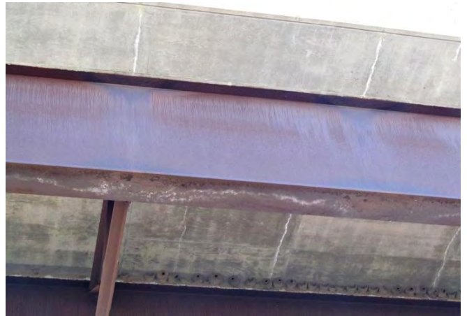
Figure 2. Exterior of west fascia girder on southbound bridge showing localized patina deterioration on all surfaces beneath cracks.
