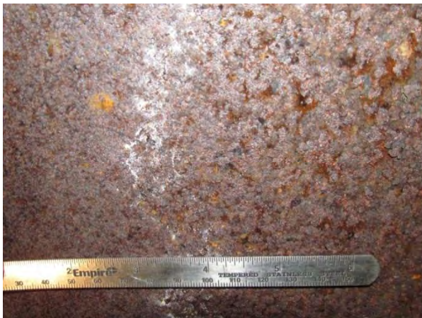
Figure 5. Close-up of discoloration and flaking on bottom flange adjacent to staining, Index = 2.
