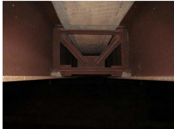
Figure 4. Typical K-brace cross-frame with bird droppings on girder bottom flanges.
