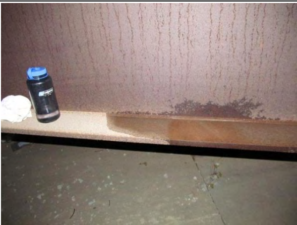
Figure 5. Poultice on east fascia interior side (not flaky). Washed with water and blotted dry.
