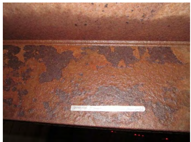
Figure 6. Washing after hand brushing of poutlice: Cleaner, but delaminated patina remains.
