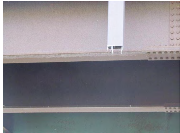
Figure 6. Fascia problems continue over main span.
