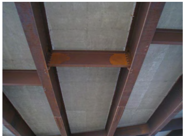
Figure 6. Areas of underdeveloped patina due to spill during construction or mill scale (Index=5).
