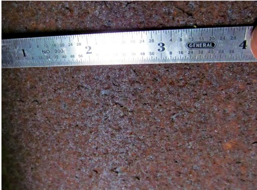
Figure 18. Close-up photo of Category 3 patina on bottom of interior girder web. Texture is less uniform but still generally adherent, with some small loose flakes.
