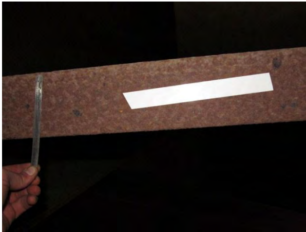
Figure 3. Index = 2 patina on vertical face of cross-brace where tape test conducted.
