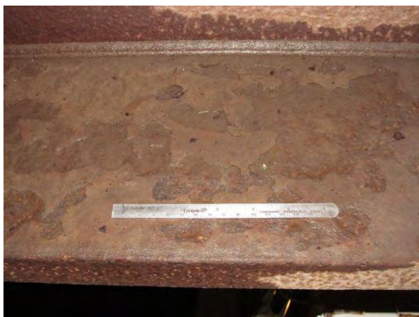
Figure 5. Washing as-is: poutlice reduced, but delamination remains.
