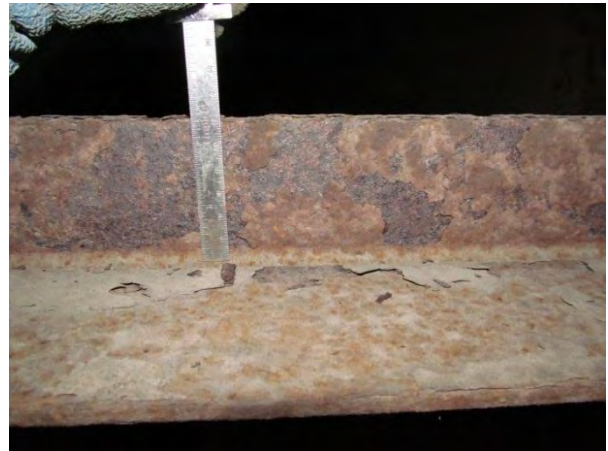
Figure 4. Heavy deterioration typical of cross-frame members over traffic lanes.
