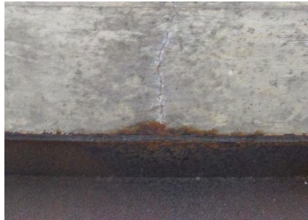
Figure 2. Top flange deterioration beneath concrete deck crack; possibly index rating of 1 on hidden top.
