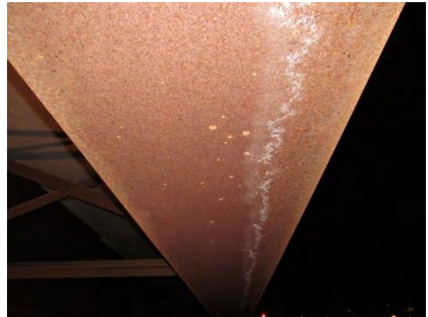
Figure 4. White staining on bottom flange of west fascia on eastbound lanes (side toward traffic).
