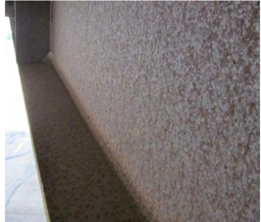
Figure 2. Typical interior web and top of bottom flange near south abutment; poutlice not flaking. Index for both surfaces is 3.
