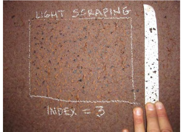
Figure 2. Interior middle of web tape test and hand scraping of loose flake (dark spots). Index later determined to be 2 based on tape flake size.
