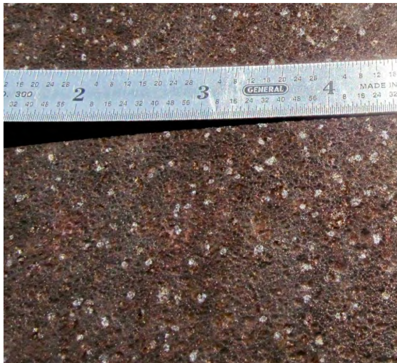
Figure 17. Close-up photo of Category 4 patina commonly observed on exterior web of fascia girder. Surface is textured but tightly adherent, and rust formations are small. No loose flakes are present.
