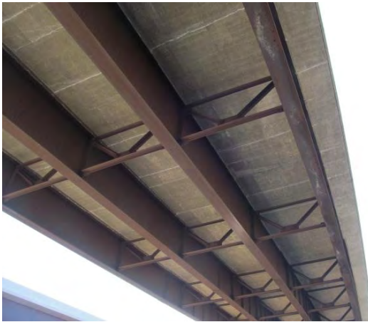
Figure 1. Typical middle bay of southbound bridge; note regular cracking with efflorescence and heavy salt staining on west fascia girder bottom flange.
