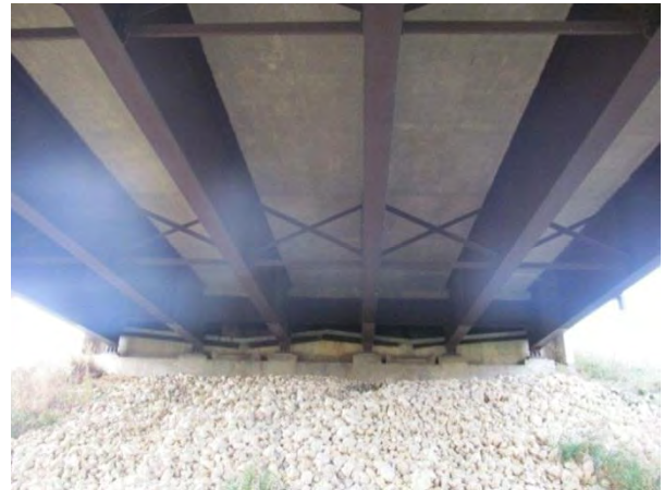
Figure 2. South abutment, showing typical cross-frames and diaphragms detailed to not stain concrete.
