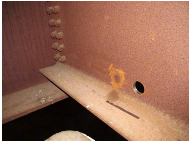
Figure 4. Heavy poutlice corrosion on diaphragm and girder flange at core location.
