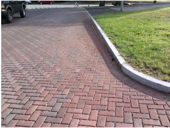
Figure 12: Run on from an intersecting pedestrian walkway.
