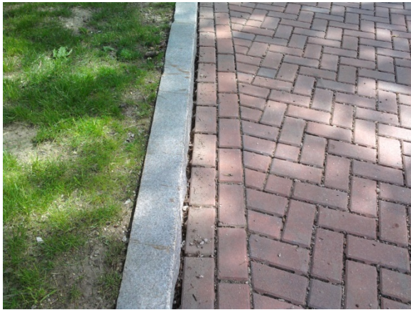
Figure 13: Loss of No. 8 stone along curb line due to erosion and cleaning.
