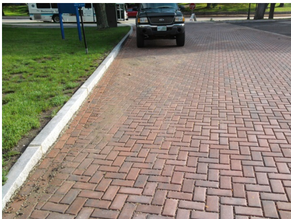
Figure 14: Another area of run on from an intersecting pedestrian walkway.
