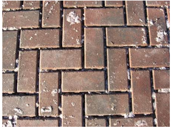
Figure 15: No. 8 joint stone has settled approximately 1 inch.
