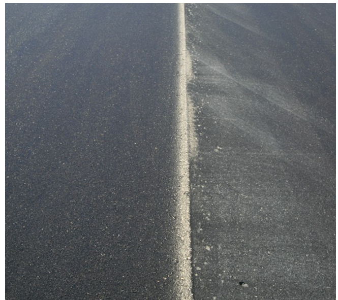
Longitudinal joint with coarse segregation
