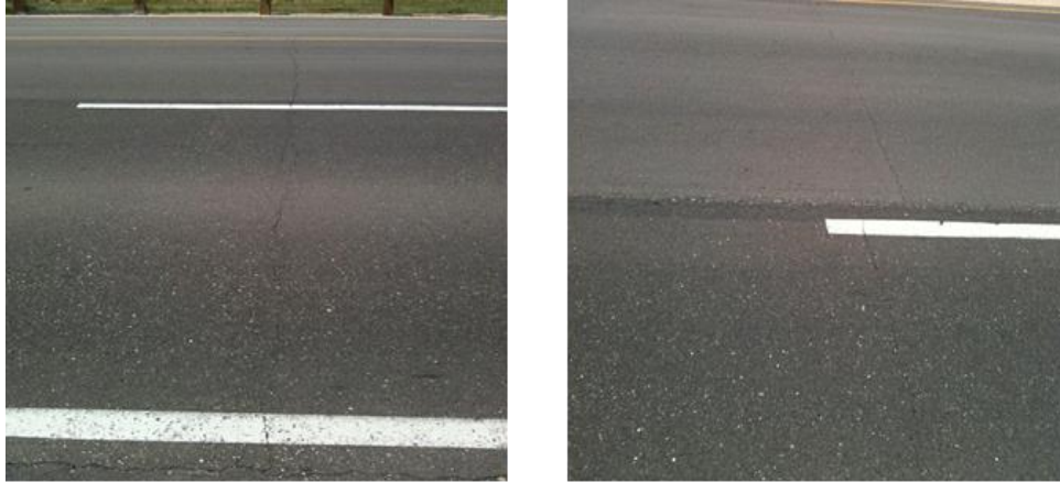
Figure 44. Longitudinal joint performance for the IA 13 project
