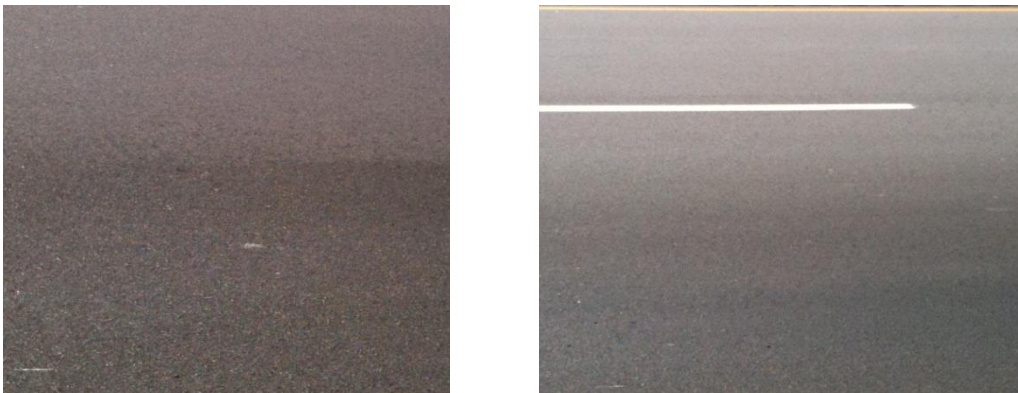
Figure 45. Longitudinal joint performance for the I-35 project
