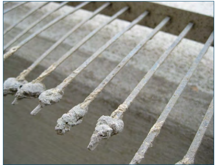
Figure 22. Excessive buildup of hardened mortar on tines
