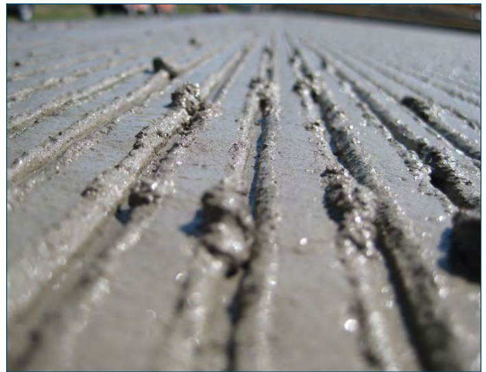
Figure 19. Redeeped mortar on the surface of the lands between the tined grooves
