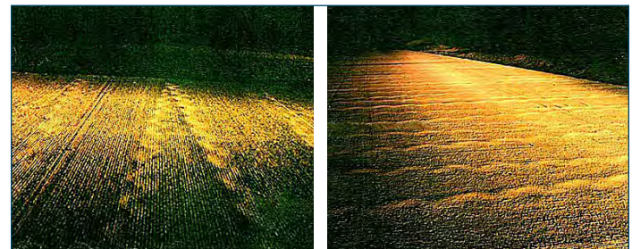
Figure 46. Unintended texture introduced by automatic longitudinal float
