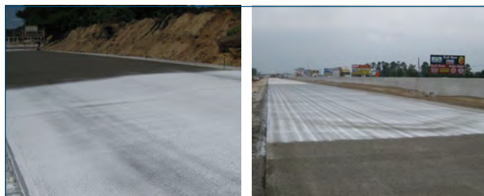
Figure 58. Poor curing practice
