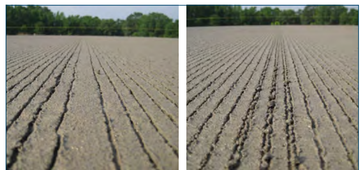
Figure 33. Poor transverse start/stop point matching – left: holiday; right: overlap
