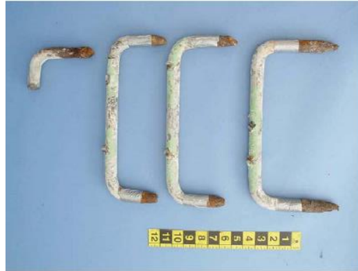
Figure 1. Corroded conditions of several U-bolt anchors that were extricated from concrete bridge barrier rail (NTSB 2010)
