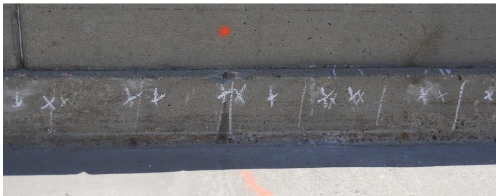
Figure 58. Suspect locations on the west end of the bridge
