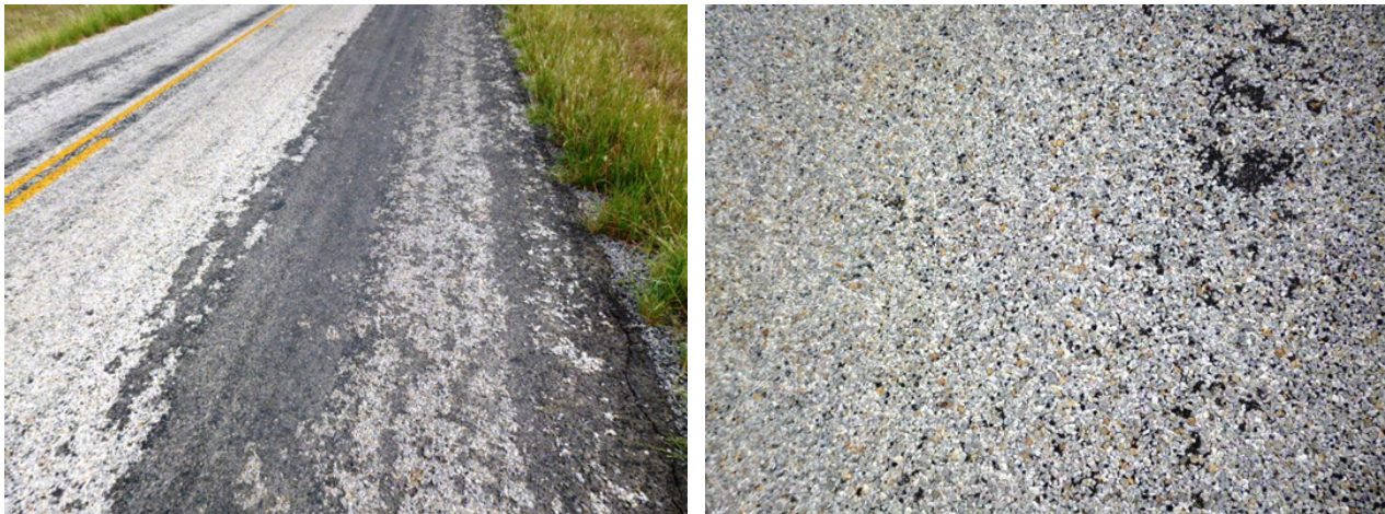
Figure 32. Example of Inadequate Performance—HS B-1.
