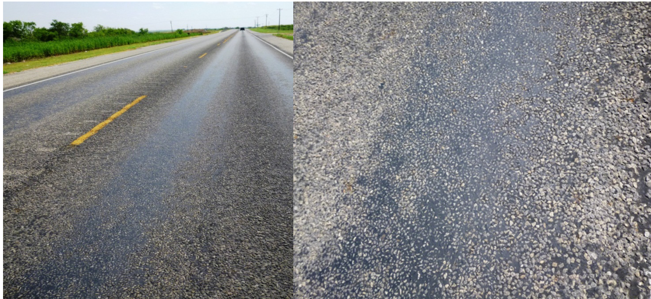
Figure 36. Example of Inadequate Performance on HS S-5.
