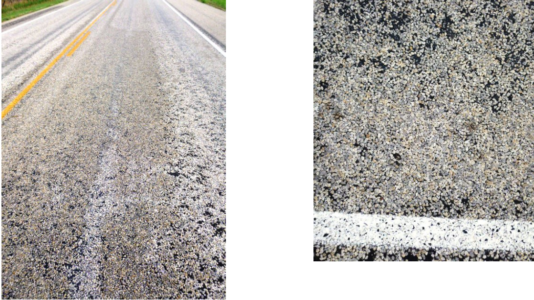
Figure 38. Example of Adequate Performance on HS B-3.
