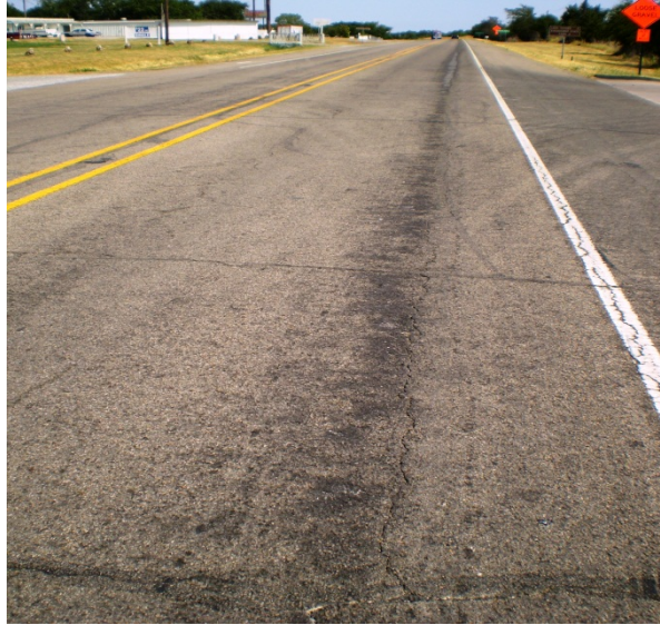
Figure 34. Example of Longitudinal and Transverse Cracks on HS P-3.
