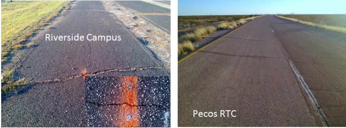
Figure A-6. Transverse Cracked Pavement Sections at Riverside Campus and Pecos RTC (by Bryan Wilson).
